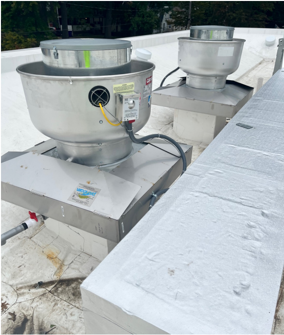
Kitchen Exhaust Fans
