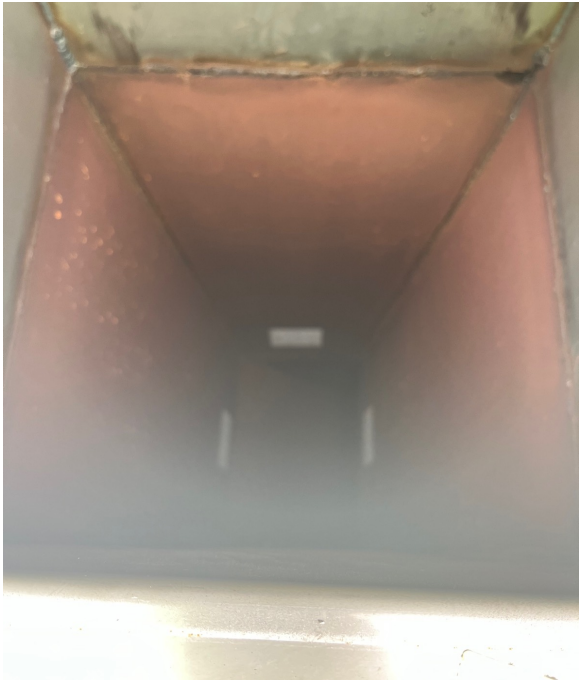
Typical Grease Duct
