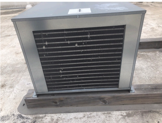
Walk-in Cooler Dirty condenser
