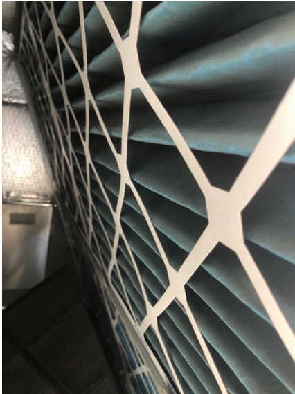
RTU-2 Dirty evaporator filters
