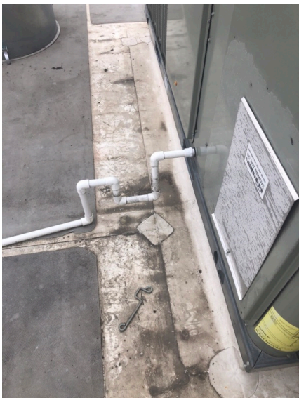
RTU-2 Condensate drain
