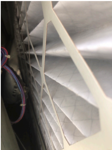
RTU-3 Clean evaporator filters
