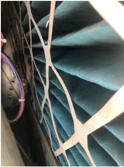
RTU-3 Dirty evaporator filters
