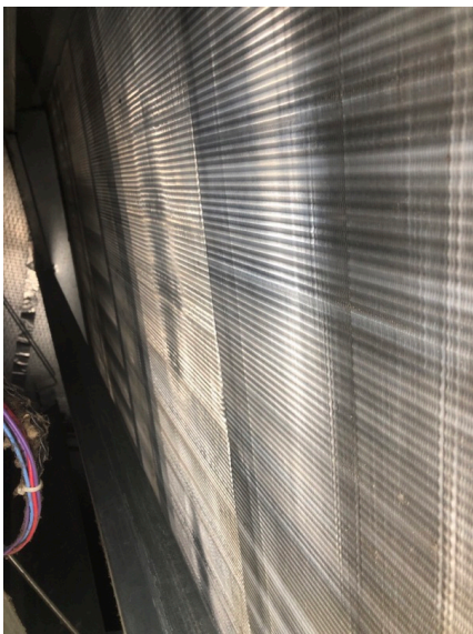
RTU-3 Dirty evaporator coil
