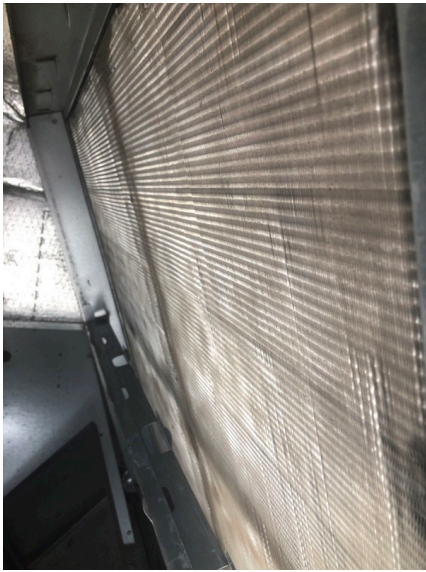
RTU-1 Dirty evaporator coil
