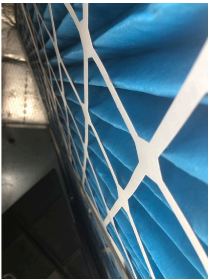
RTU-1 Clean evaporator filters
