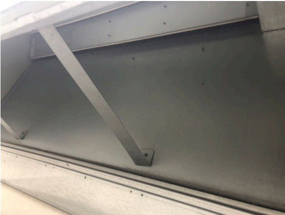
RTU-3 Dirty outside air filters
