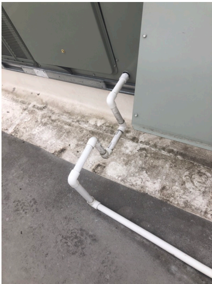
RTU-1 Condensate drain
