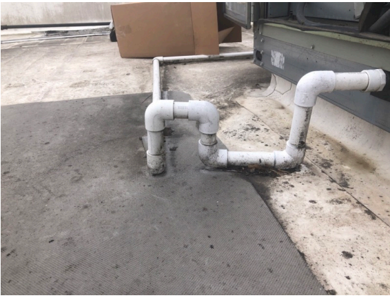
RTU-3 Condensate drain
