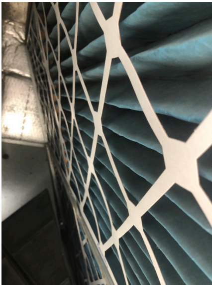
RTU-1 Dirty evaporator filters
