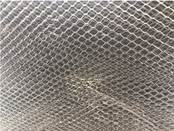
MAU Dirty outside air filters
