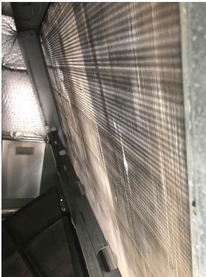
RTU-2 Dirty evaporator coil
