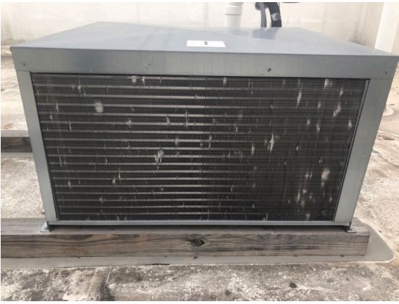
Walk-in Freezer Dirty condenser
