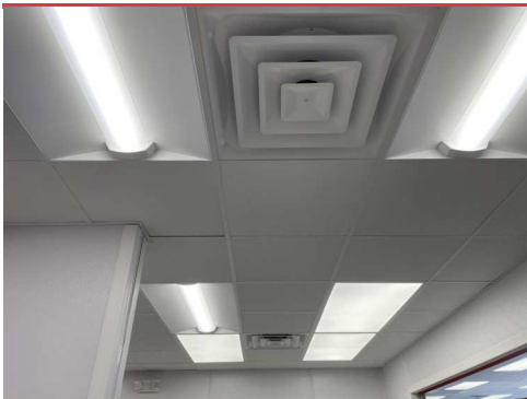
KITCHEN DIFFUSERS (TEMPORARY 4-WAYS)
