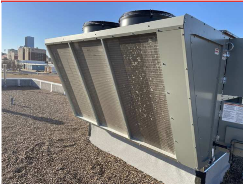
DOAS CONDENSER COIL DAMAGED
