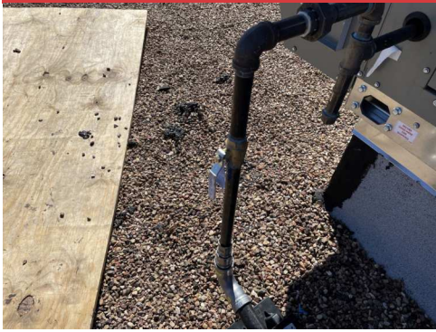
DOAS GAS VALVE OPEN
