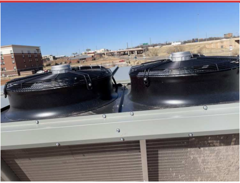
DOAS CONDENSER FANS OPERATING
