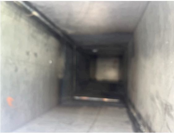
EF-1 Grease duct
