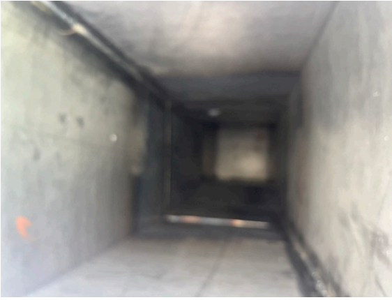
EF-1 Grease duct
