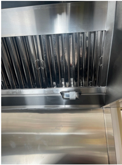
HD-1 Grease cup installed
