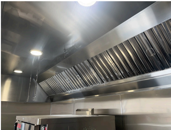
HD-1 Hood filters, lights installed and functional.
