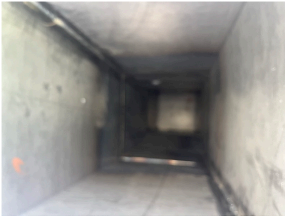
EF-1 Grease duct
