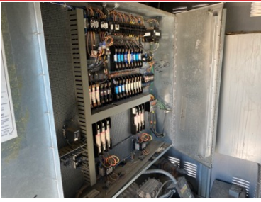
NORTH MAIN SALES RTU ELECTRICAL
