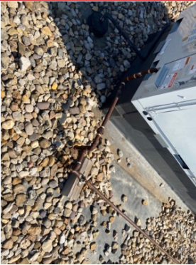
RTU7 GAS VALVE POSITION
