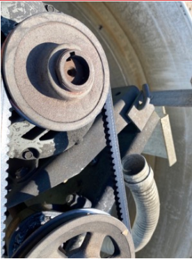
LEFT DELI HOOD EF8A Belt starting to crack
