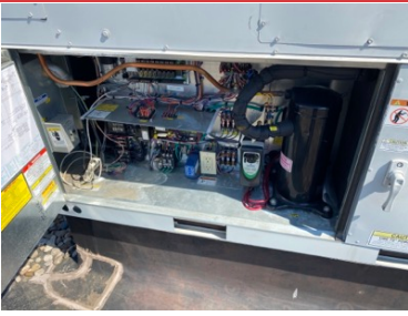
RTU3 ELECTRIC SECTION
