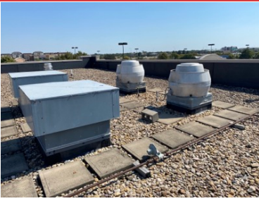
EF8 & 8A W/ SF1 & 2 DELI HOOD EXHAUST AND SUPPLY FANS
