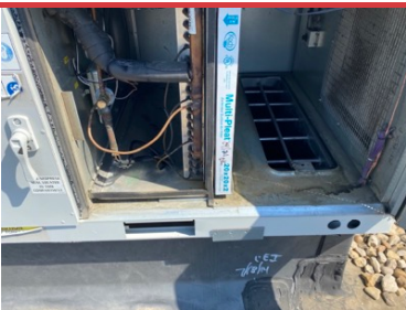
RTU6 FILTER SECTION
