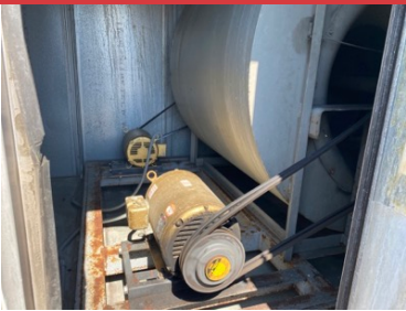
NORTH MAIN SALES RTU FAN SECTION
