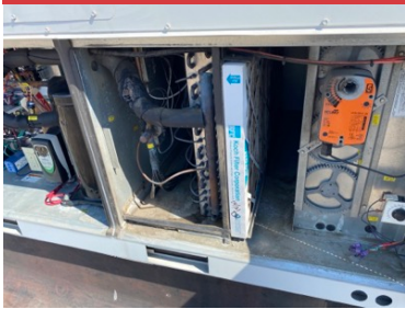
RTU3 FILTER SECTION
