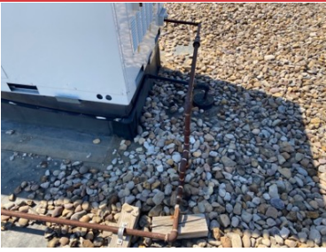
RTU6 GAS VALVE POSITION
