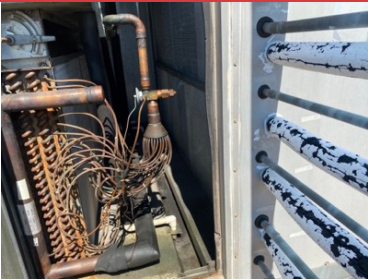
NORTH MAIN SALES RTU EVAPORATOR SECTION
