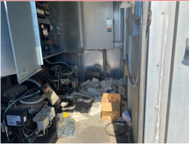
NORTH MAIN SALES RTU ELECTRICAL VESTIBULE
