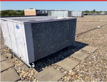
RTU4 CONDENSER FINS Damaged
