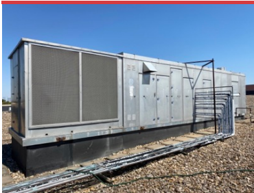
RTU1 NORTH MAIN SALES
