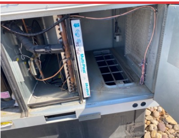
RTU7 FILTER SECTION
