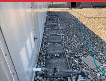
NORTH MAIN SALES RTU DRAINS
