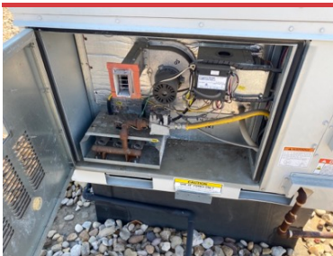
RTU3 HEAT SECTION
