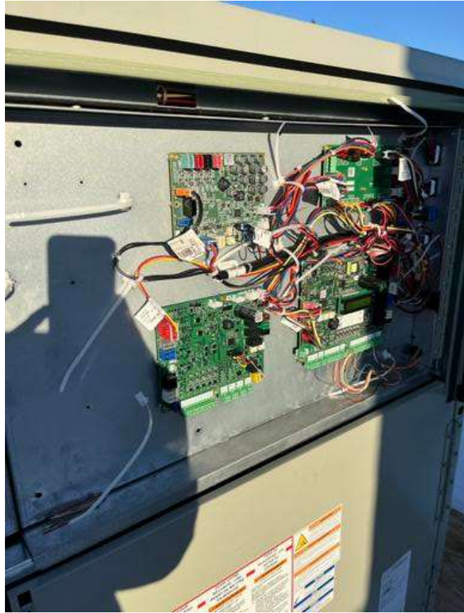
Missing Delay Timer and Temperature Controller
