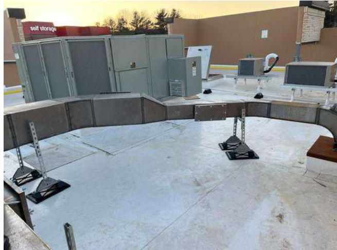
Grease Duct Supports
