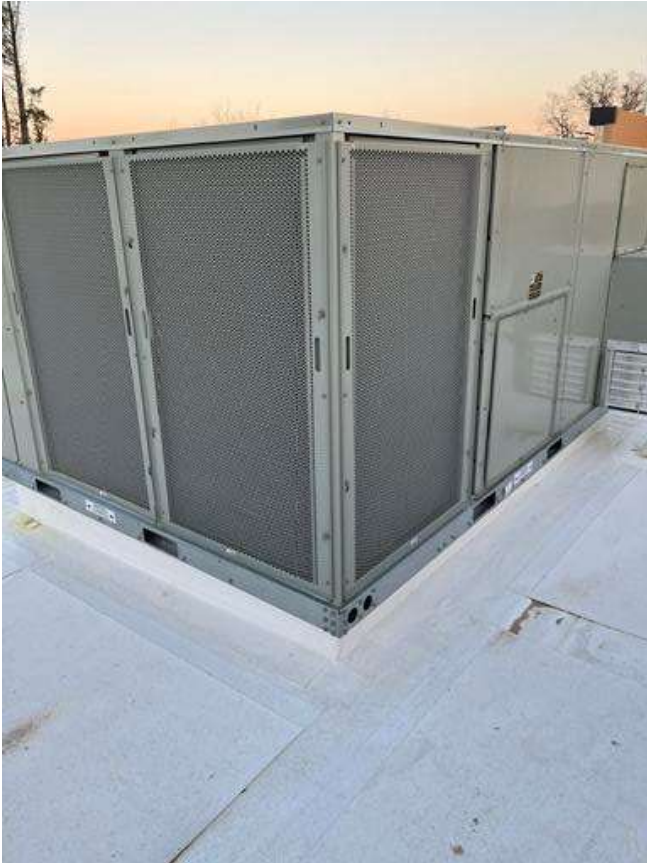
Missing Seismic Clips
