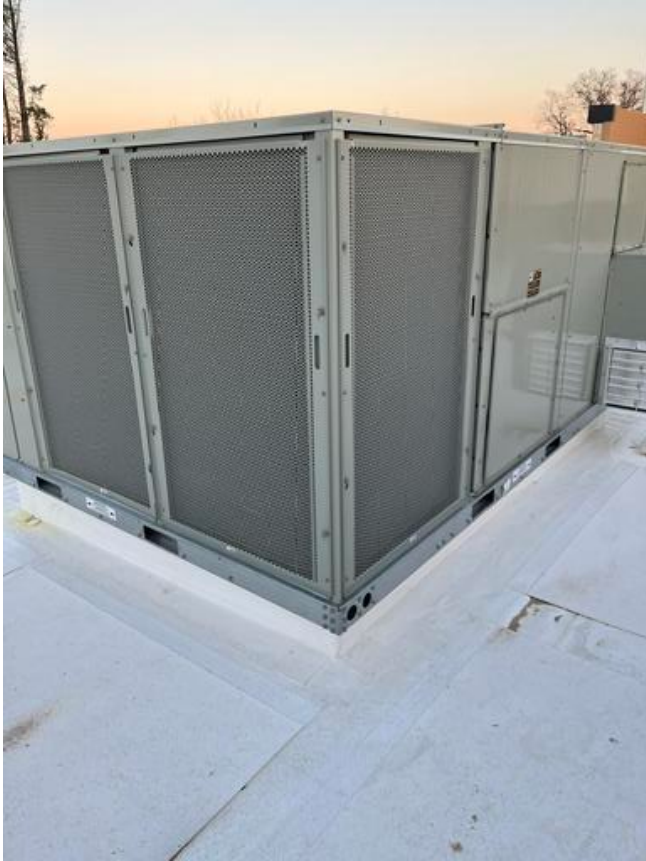
Missing Seismic Clips
