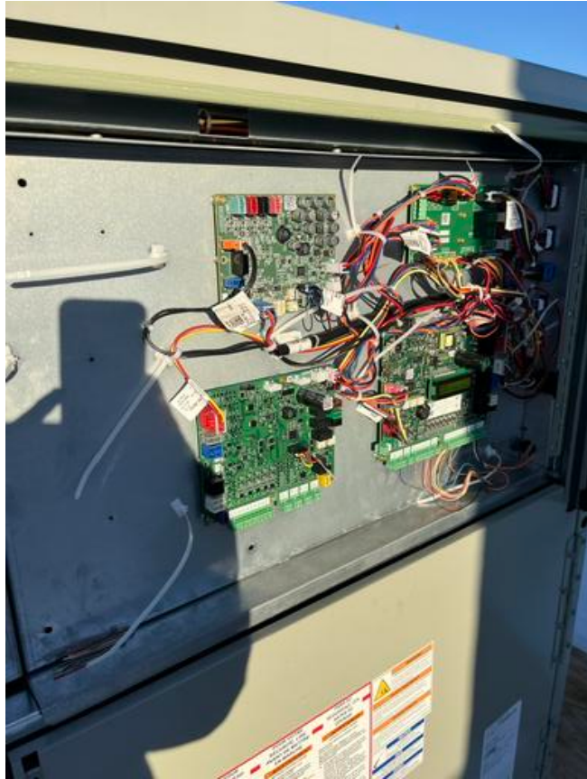
Missing Delay Timer and Temperature Controller
