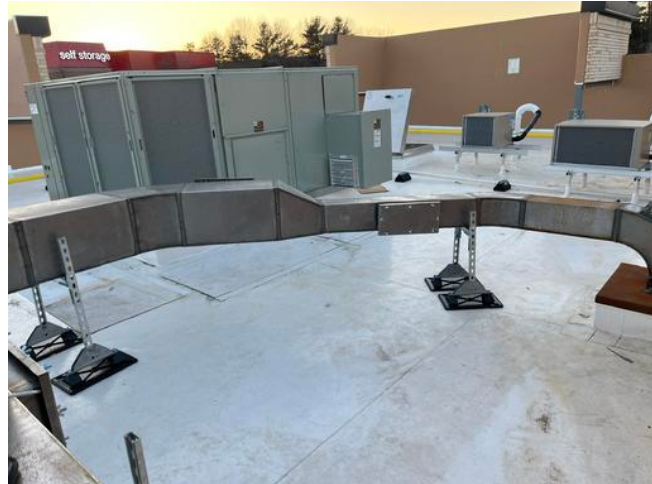
Grease Duct Supports
