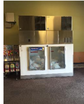
ICE MACHINE IN VESTIBULE
