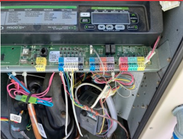
RTU 2 CONTROLS WIRING
