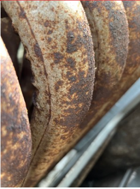
RTU 1 HEAT EXCHANGER TUBES RUSTY
