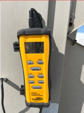
RTU 2 RETURN Dining Unit
