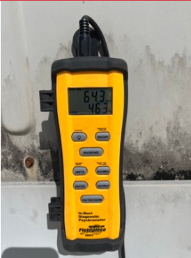
RTU 1 DISCHARGE Kitchen Unit
