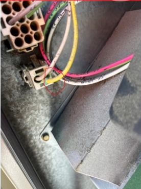
DINING RTU DAMAGED WIRE
