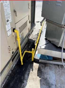
GAS LINES PAINTED
