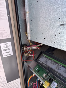
DINING RTU DAMAGED WIRE
