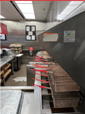
KITCHEN HOOD & EQUIPMENT
