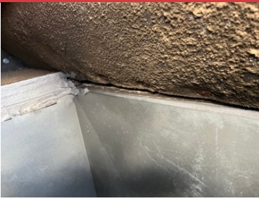
DINING RTU SUPPLY DROP
