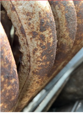
RTU 1 HEAT EXCHANGER TUBES RUSTY
