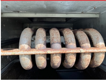
RTU 1 HEAT EXCHANGER TUBES
