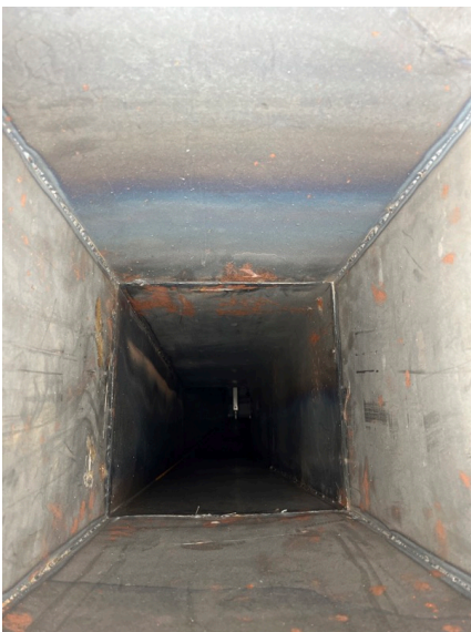
PRV-3 Grease duct
