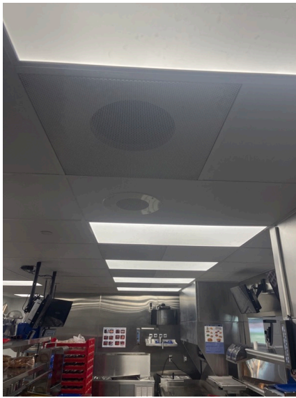
RTU-2 Cookline diffusers perforated.
