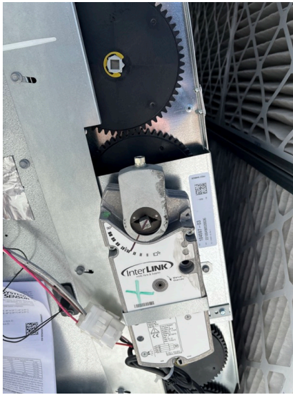
RTU-2 OA damper position marked
