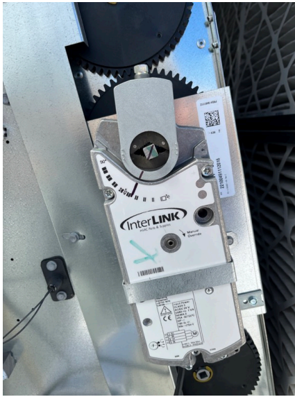
RTU-1 OA damper position marked
