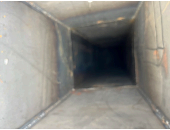
PRV-2 Grease duct
