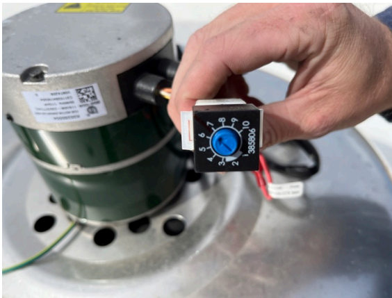
PRV-1 Setpoint marked
