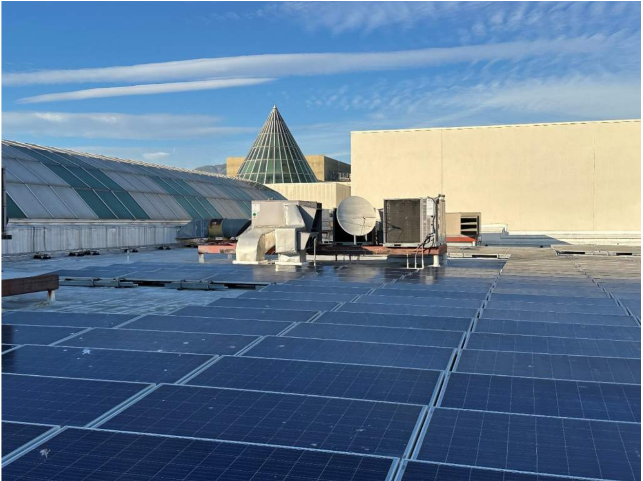
Photograph 4 – Overall view of units on rooftop concealed from line of site and centrally located on the roof
