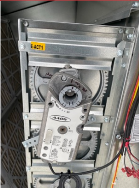
RTU1 MINIMUM DAMPER POSITION
