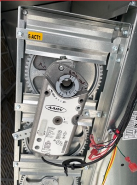
RTU2 MINIMUM DAMPER POSITION
