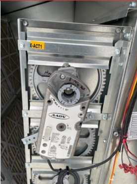
RTU1 MINIMUM DAMPER POSITION
