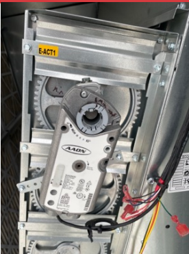
RTU2 MINIMUM DAMPER POSITION
