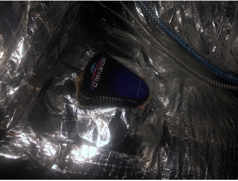
AHU-2 REME HALO
