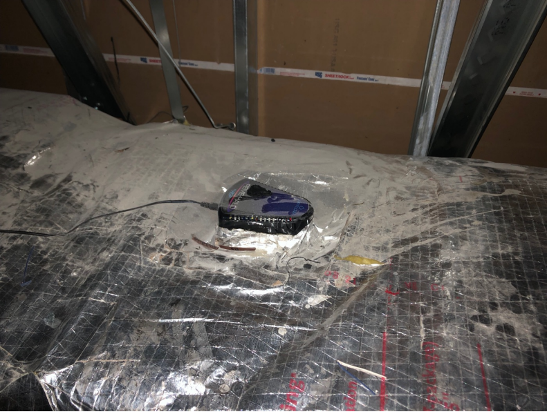
AHU-3 REME HALO
