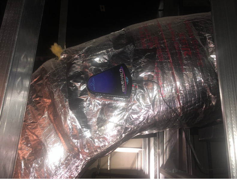
AHU-1 REME HALO
