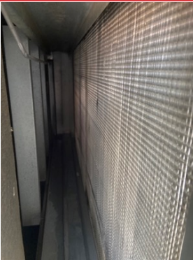
RTU-1 EVAP COIL CLEAN
