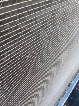
RTU-2 CONDENSER CLEAN
