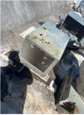
WALK-IN COOLER CONDENSER DIRTY
