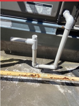
RTU-1 CONDENSATION DRAIN CLEAN
