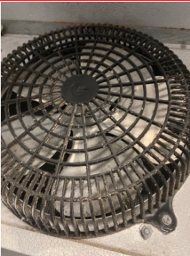
FANS NOT RUNNING WALK IN COOLER
