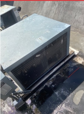
WALK IN FREEZER CONDENSER DIRTY
