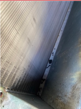
RTU-2 CONDENSATION TRAY CLEAN
