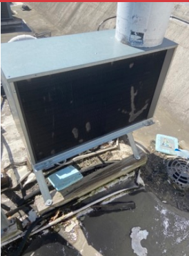
SODA MACHINE CONDENSER DIRTY
