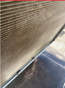
RTU-3 CONDENSER CLEAN
