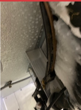
ICE BUILD UP ON PEN PIPE
