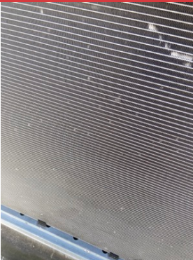
RTU-1 CONDENSER DIRTY
