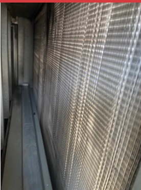
RTU-2 EVAP COIL CLEAN
