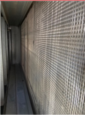
RTU-1 EVAP COIL DIRTY
