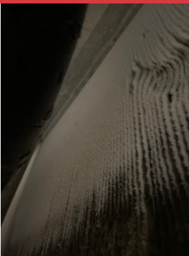
ICE ON COILS WALK IN COOLER
