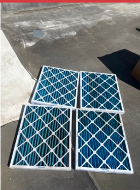
RTU-3 EVAP FILTER DIRTY
