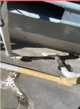
RTU-2 CONDENSATE DRAINE Snapped drain
