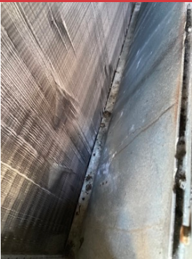
RTU-3 CONDENSATION TRAY CLEAN
