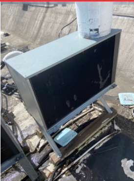
SODA MACHIN CONDENSER CLEAN
