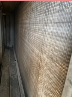
RTU-3 EVAP COIL CLEAN
