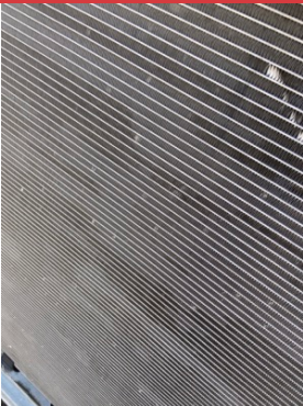
RTU-1 CONDENSER CLEAN
