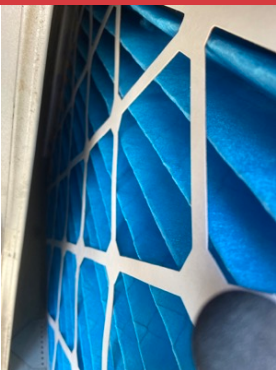
RTU-1 EVAP FILTER CLEAN
