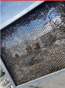
MAU OA FILTERS NEED TO BE REPLACED
