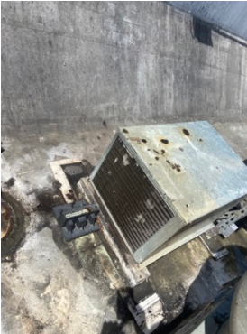
WALK-IN COOLER CONDENSER CLEAN
