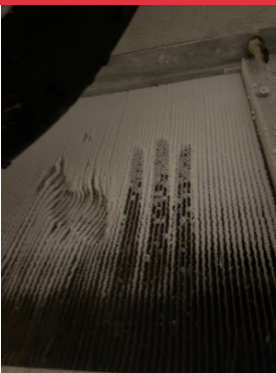
WALK IN COOLER DIRTY
