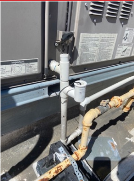
RTU-3 CONDENSATION DRAIN CLEAN
