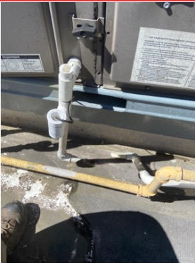
RTU-2 CONDENSATION DRAIN CLEAN
