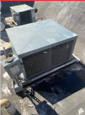
WALK IN FREEZER CONDENSER DIRTY
