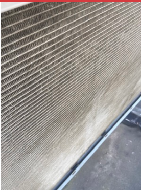
RTU-3 CONDENSER DIRTY
