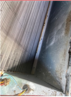
RTU-1 CONDENSATION TRAY CLEAN
