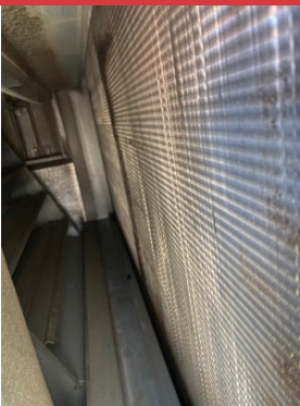
RTU-2 EVAP COIL DIRTY
