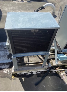
ICE MACHINE CONDENSER DIRTY
