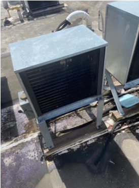
ICE MACHINE CONDENSER CLEAN
