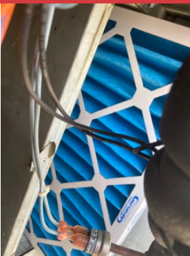
RTU-3 EVAP FILTER CLEAN
