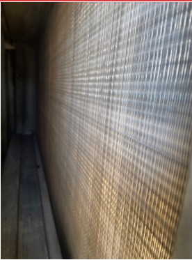
RTU-3 EVAP COIL DIRTY
