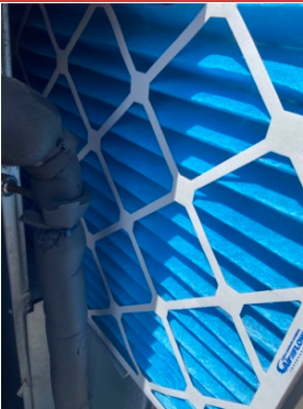
RTU-1 EVAP FILTER CLEAN
