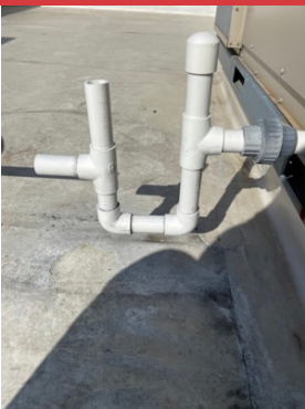
RTU-1 CONDENSATION DRAIN
