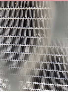
RTU-1 CONDENSER COIL DIRTY
