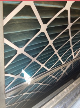
RTU-1 EVAP FILTERS DIRTY
