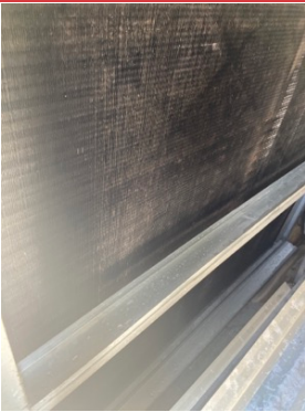
RTU-1 EVAP COIL CLEAN
