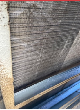
RTU-3 EVAP COIL CLEAN
