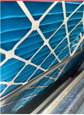
RTU-2 EVAP FILTERS CLEAN
