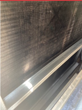
RTU-1 EVAP COIL DIRTY
