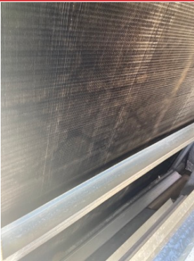
RTU-2 EVAP COIL DIRTY
