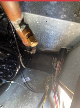
RTU-2 DRAIN PAN CLEAN
