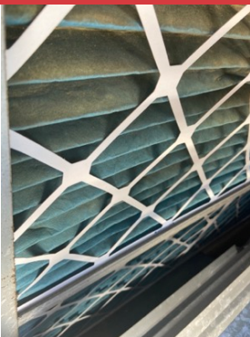
RTU-2 EVAP FILTER DIRTY
