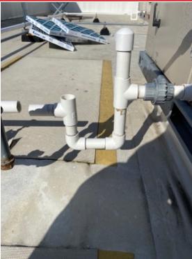
RTU-2 CONDENSATION DRAIN
