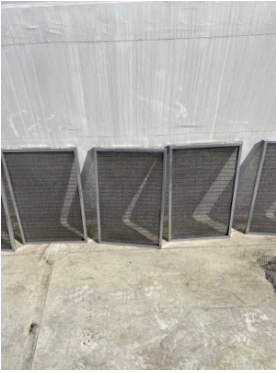
RTU-2 OA FILTER CLEAN
