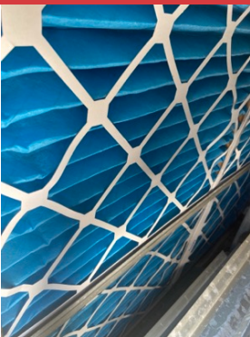
RTU-1 EVAP FILTERS CLEAN
