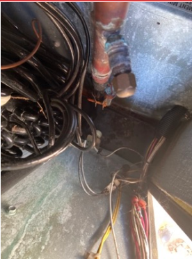
RTU-1 DRAIN PAN CLEAN
