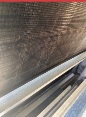
RTU-2 EVAP COIL CLEAN
