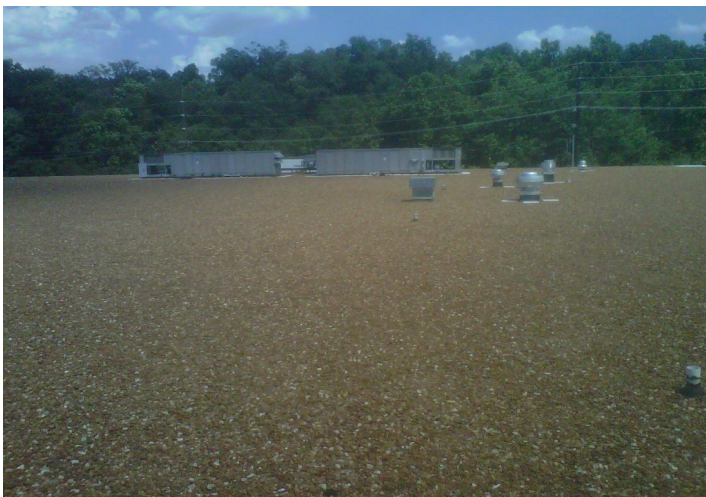
rtu-1 on left, rtu-2 on right
