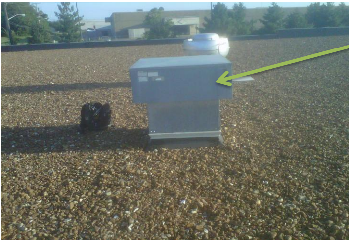
mua suppls fryers and stove oven unit not running - fix if plan on using existing system.
