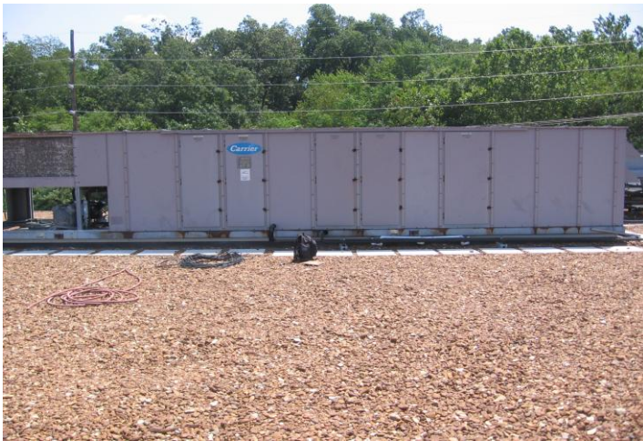
rtu-1 and rtu-2
