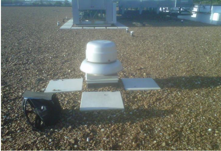
fan not in use over by bakery - Could be Capped if not used.
