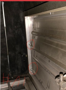
AHU-1 OA DAMPER STOPPED BY SELF TAPPING SCREWS
