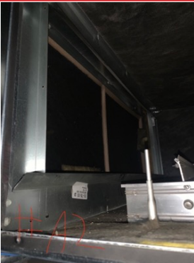
AHU-2 FILTERS ARE EXTREMELY DIRTY
