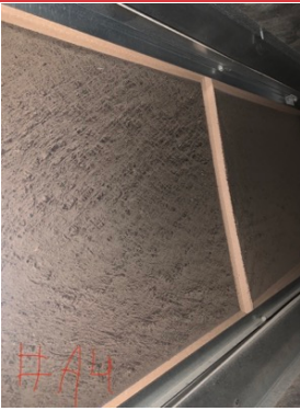
AHU-4 FILTERS ARE DIRTY
