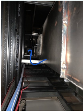
SECOND DOOR PICTURED LOOKS LOOSE
