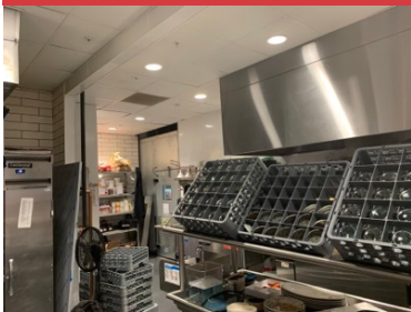
BOH HOOD-1 ON LEFT AND DISH HOOD ON RIGHT
