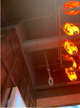
DUCTWORK IN DINING IS 20' ISH OF THE GROUND
