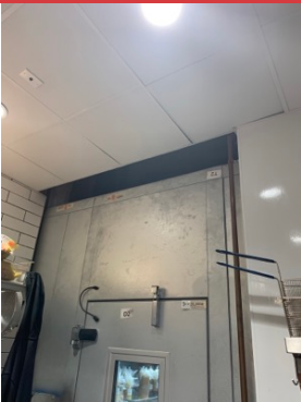
CEILING NOT SEALED TO WALK-IN COOLER.
