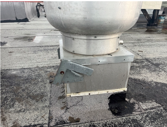
EF-1 Hinge broken, not secured
