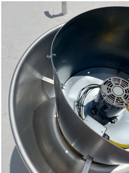
PRV-3 Dent in fan housing.
