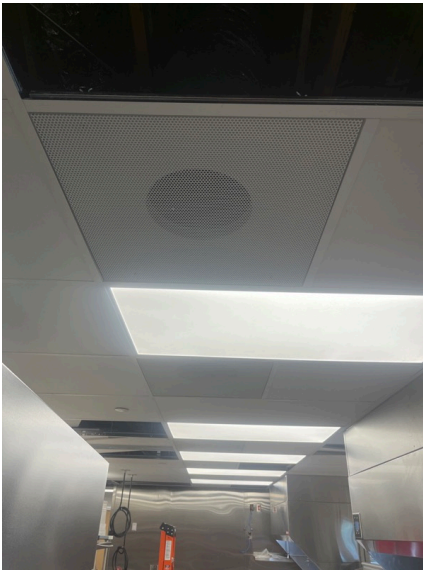
RTU-2 Cookline diffusers perforated.
