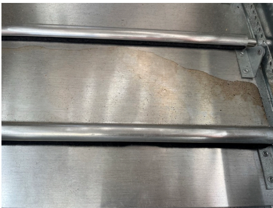
PRV-1 Backdraft damper installed and able To move freely.
