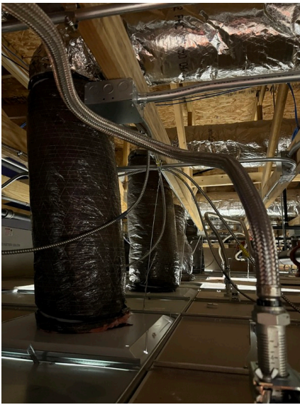
RTU-2 Cool line diffuser installation correct
