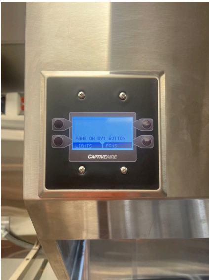
Captive Air Hood HMI
