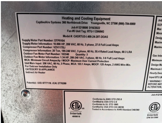
RTU-1 Unit label
