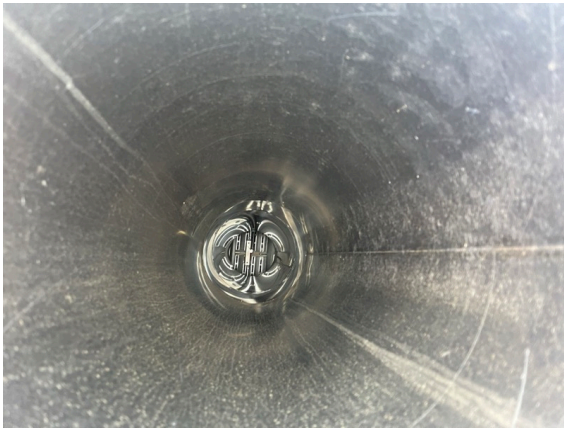
PRV-2 Grease duct
