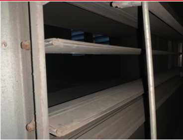
UNIT DAMPER AND OA INTAKE LOUVERS
