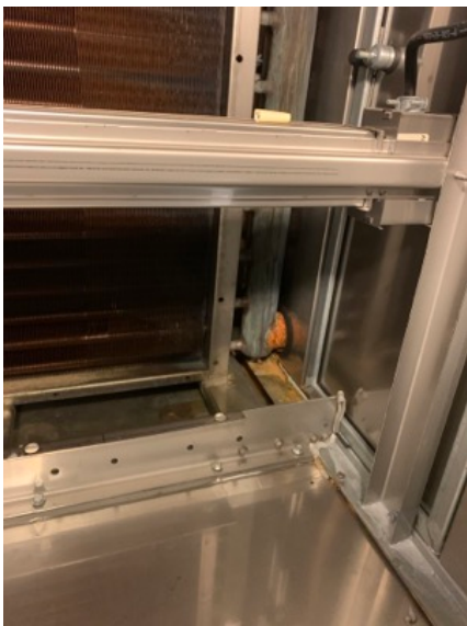
CORROSION ON COIL INLET
