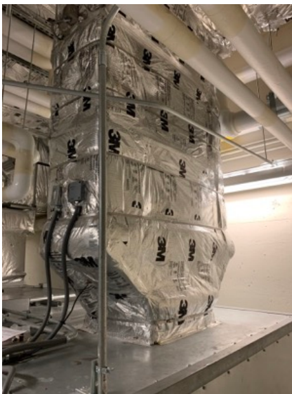
UNABLE TO TRAVERSE SUPPLY DUCT DUE TO SOUND ATTENUATION
