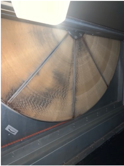
HEATING WHEEL There is a little bit of damage
