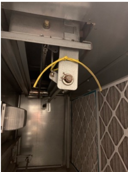
RETURN DAMPER SECURED WITH WIRE TIE
