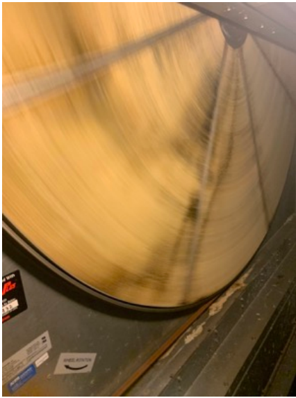
S1- Heating Wheel
