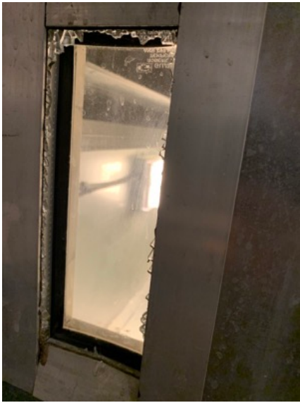
BROKEN WINDOW ON RETURN PLENUM DOOR
