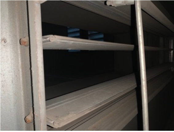
UNIT DAMPER AND OA INTAKE LOUVERS
