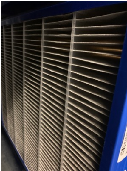
FINAL FILTER CONDITION
