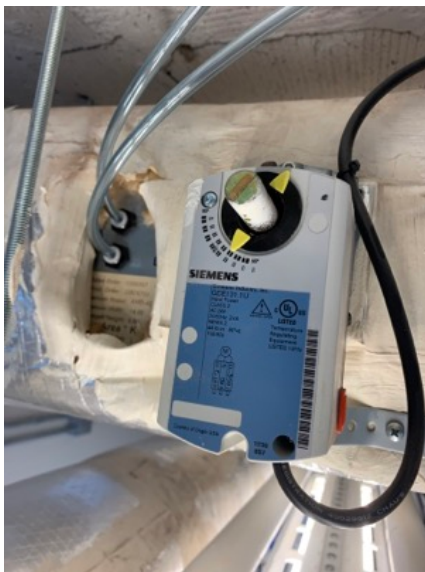
DAMPER POSITION APPROXIMATELY 50%
