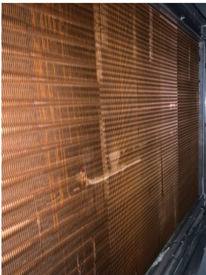
SLIGHT DAMAGE TO COOLING COIL. NO MORE THAN 5% OF COIL IS DAMAGED
