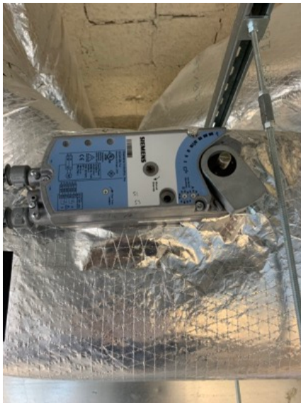
OA DAMPER POSITION DURING TESTING
