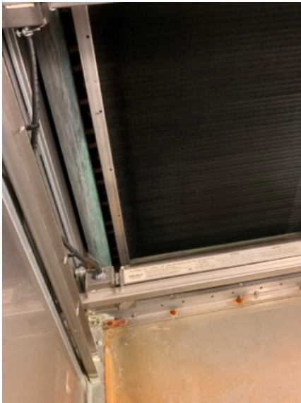
MINOR CORROSION ON COOL COIL
