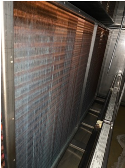
OXIDATION ON COIL
