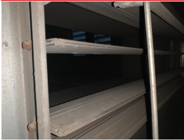
UNIT DAMPER AND OA INTAKE LOUVERS
