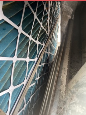
RTU-2 EVAP FILTER DIRTY
