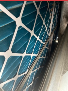
RTU-1 EVAP FILTER DIRTY
