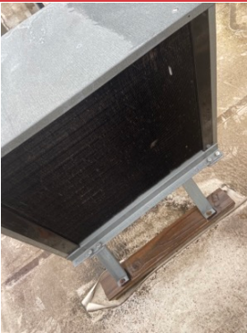
ICE MACHINE CONDENSER DIRTY
