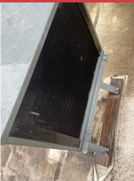
ICE MACHINE CONDENSER CLEAN
