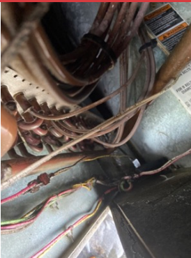
RTU-3 CONDENSATION TRAY CLEAN
