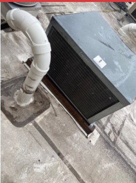
WALK IN FREEZER CONDENSER DIRTY
