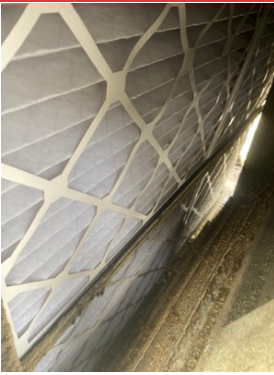
RTU-3 EVAP FILTER CLEAN
