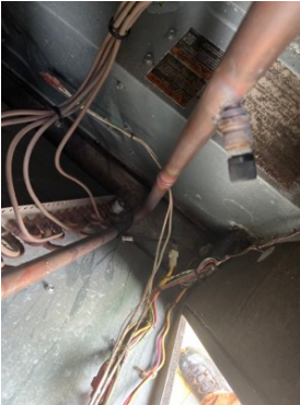
RTU-1 CONDENSATION TRAY CLEAN
