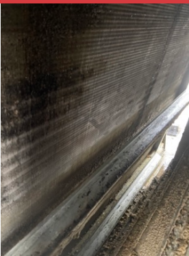
RTU-3 EVAP COIL CLEAN
