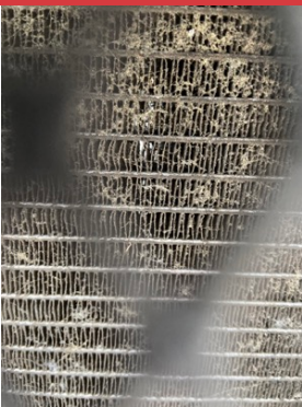
RTU-3 CONDENSER DIRTY
