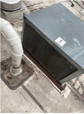
WALK IN FREEZER CONDENSER DIRTY
