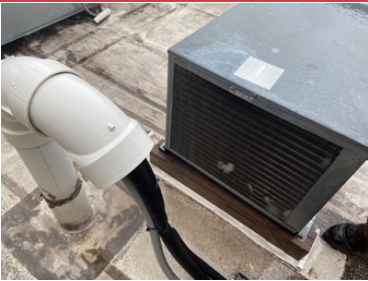
WALK-IN COOLER CONDENSER DIRTY
