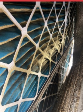
RTU-3 EVAP FILTER DIRTY
