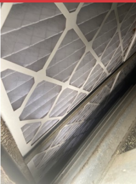
RTU-1 EVAP FILTER CLEAN
