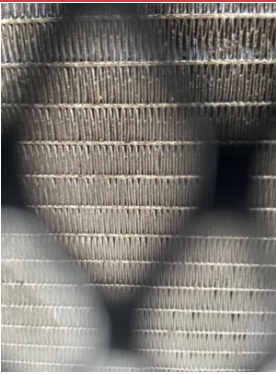
RTU-1 CONDENSER CLEAN
