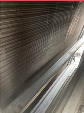
RTU-1 EVAP COIL DIRTY
