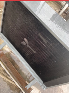
SODA MACHINE CONDENSER DIRTY
