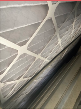
RTU-1 EVAP FILTER CLEAN
