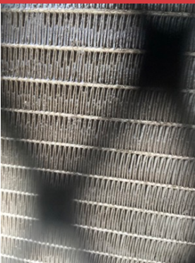
RTU-2 CONDENSER CLEAN
