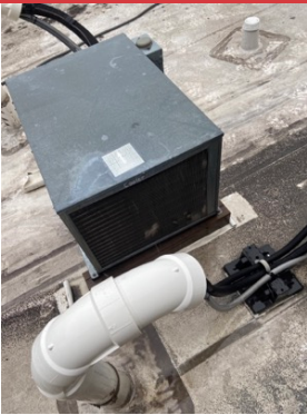
WALK-IN COOLER CONDENSER CLEAN
