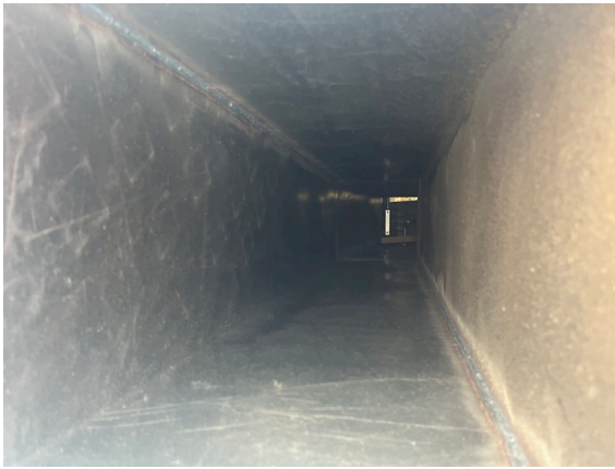
PRV-3 Grease duct
