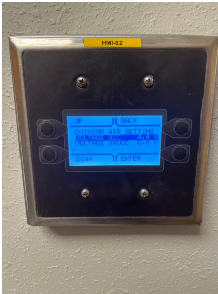
RTU-1 OA Damper Position Marked
