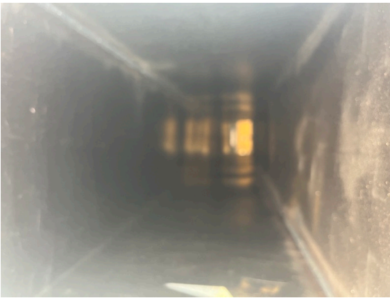
PRV-2 Grease duct
