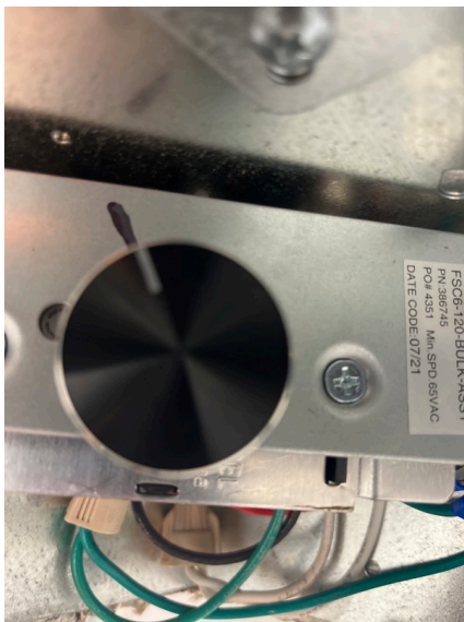
EF-1A Speed controller marked. Set to max.
