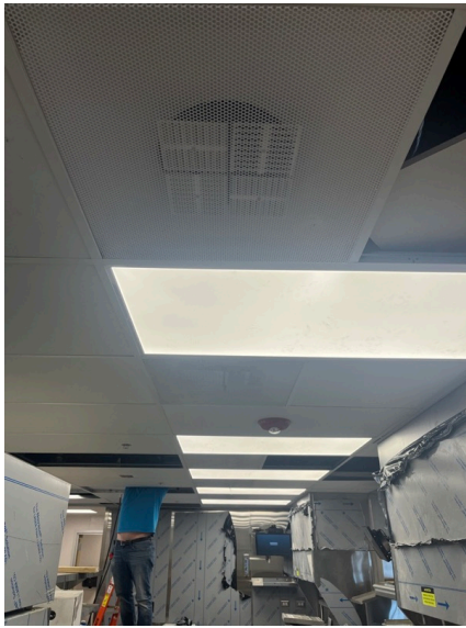
RTU-2 Cookline diffusers perforated.
