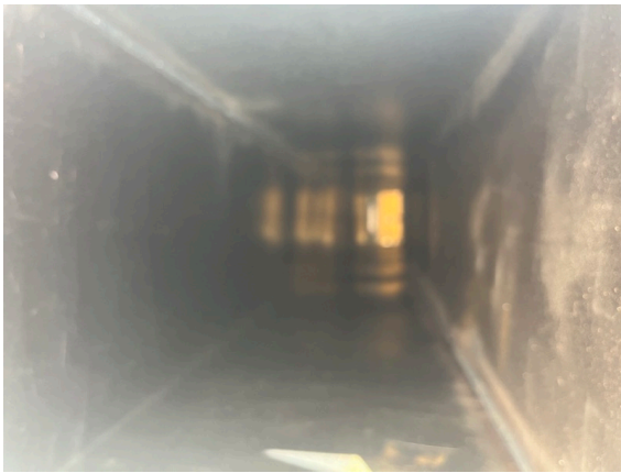
PRV-2 Grease duct
