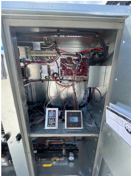
RTU-2 Control wiring
