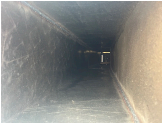
PRV-3 Grease duct
