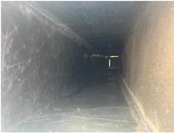
PRV-3 Grease duct
