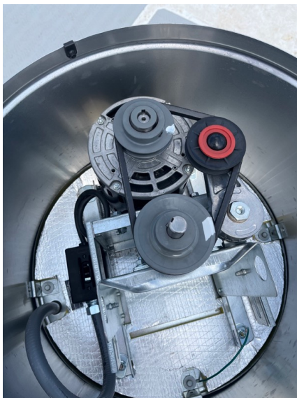
PRV-3 Disconnect installed.
