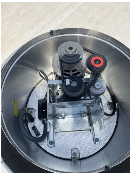
PRV-2 Disconnect installed.
