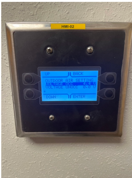
RTU-1 OA Damper Position Marked
