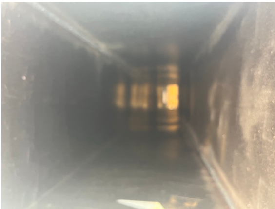
PRV-2 Grease duct
