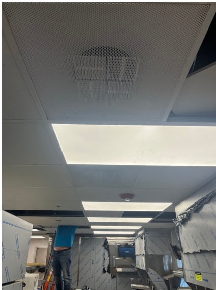
RTU-2 Cookline diffusers perforated.
