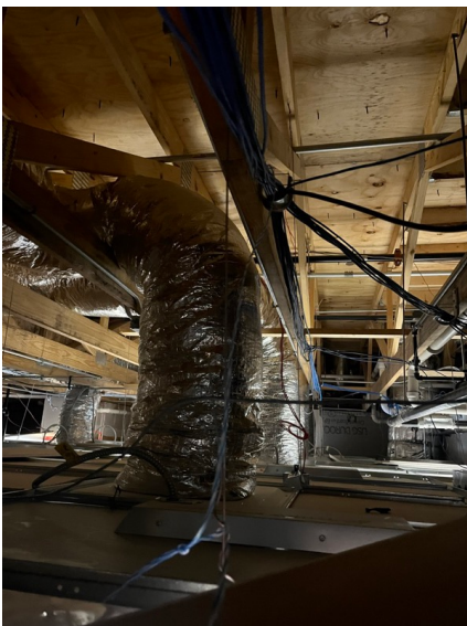
RTU-2 Cookline diffuser drops.
