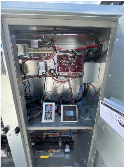
RTU-2 Control wiring
