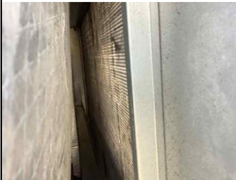
Name: Are the condenser coils free of damage and clean? .jpg Captured: 8/11/2021 1:58 PM Caption:
