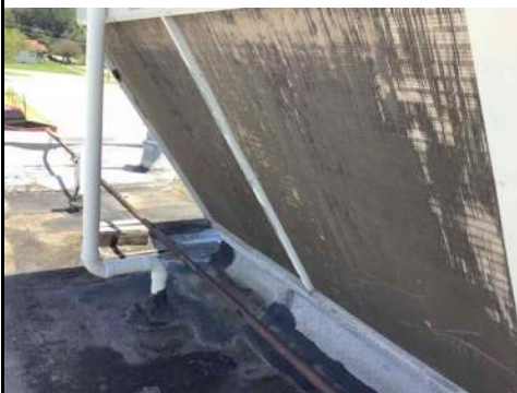
Name: Are the evaporator coils free of damage and clean?.jpg Captured: 8/11/2021 1:53 PM Caption:
