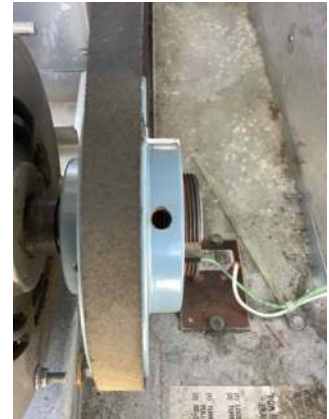
Name: Unit is over amping and could not be slowed down d.jpg Captured: 8/11/2021 3:18 PM
