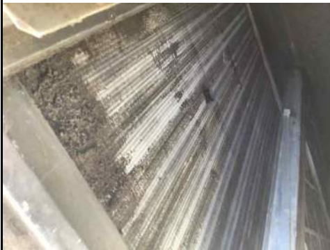
Name: Are the condenser coils free of damage and clean? .jpg Captured: 8/11/2021 1:24 PM Caption:
