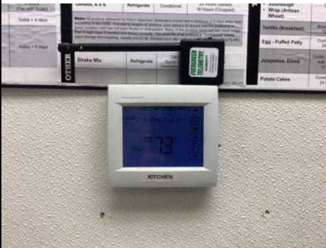
Name: Kitchen TStat.jpg Captured: 8/23/2021 10:16 AM Caption:
