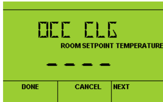
Set occupied cooling setpoint [nciTempSetpoints, occupiedCool]
