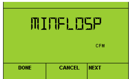
Minimum airflow setpoint at calibration [nciBalanceSetPts, MinMeasFlowSpt]
