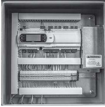
Programmable Logic Controller (PLC) Control Box (1 per fan system)
