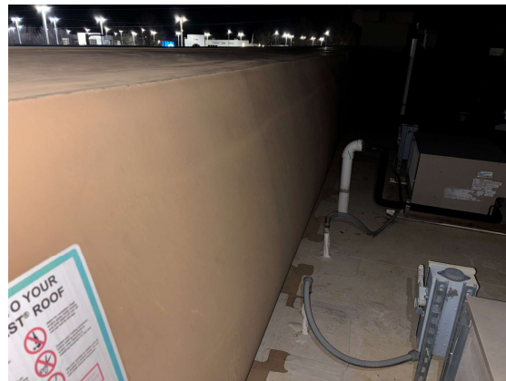
Figure 32. Roof material on parapet blowing out during pressurization test. Link to video:
