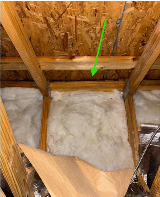
Figure 1. Typical area where leakage was observed along exterior walls
