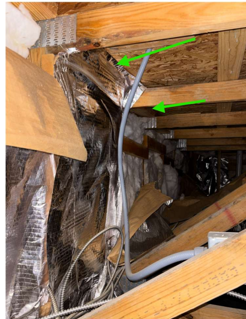
Figure 2. Typical area where leakage was observed along exterior walls
