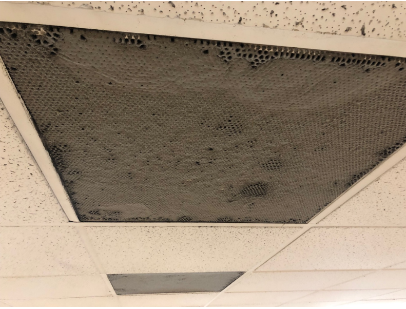
RTU-5 RETURN GRILLES NEAR DELI ARE VERY DIRTY.
