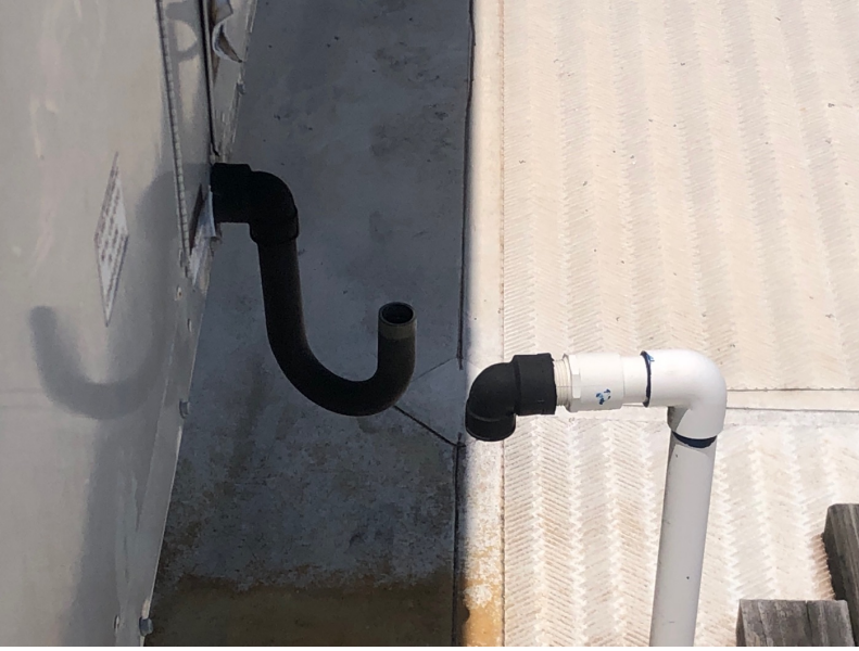
NEARLY ALL CONDENSATE P TRAPS DISCONNECTED FROM ROOFTOP DRAINS.
