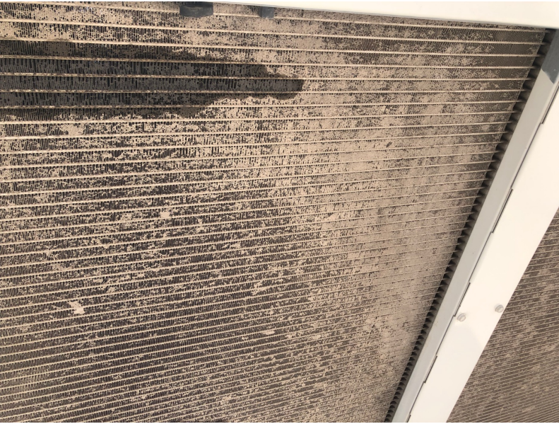
RTU-6, 10, 12, 15, 22 HAVE DIRTY CONDENSER COILS.
