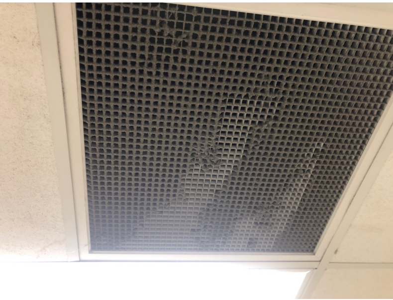
PERIMETER UNIT RETURN GRILLES DIRTY.
