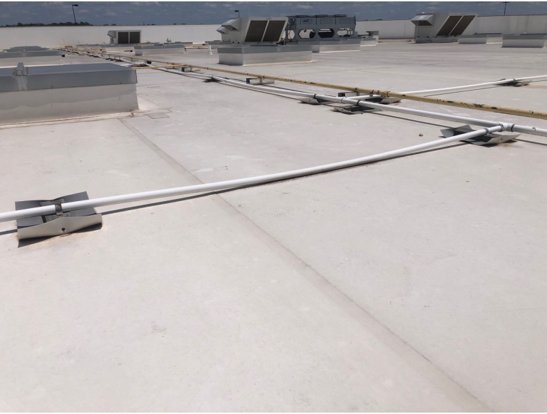
SAGS PRESENT IN ROOFTOP CONDENSATE DRAINS.
