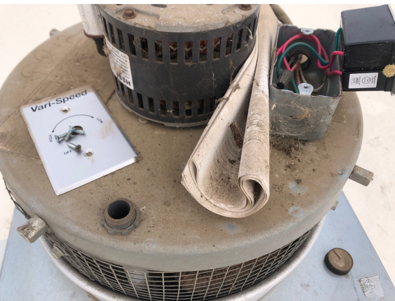
EF-S OUT OF COMMISSION. NO POWER RUN TO UNIT. WASP NESTS BUILT ALONG FAN WHEEL.
