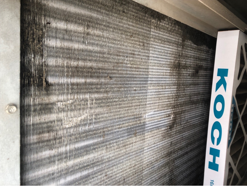
RTU-2 AND 15 HAVE MODERATELY DIRTY EVAPORATOR COILS.
