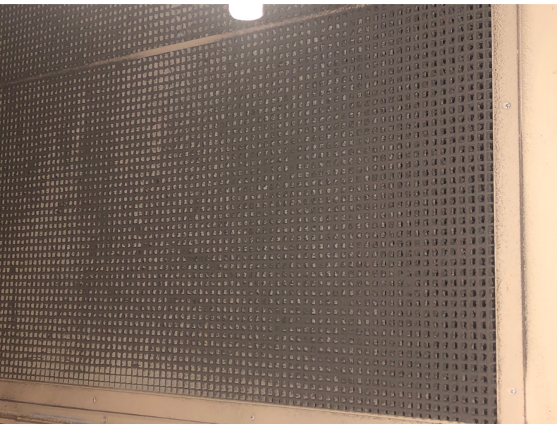
SALES FLOOR UNIT RETURN GRILLES DIRTY.
