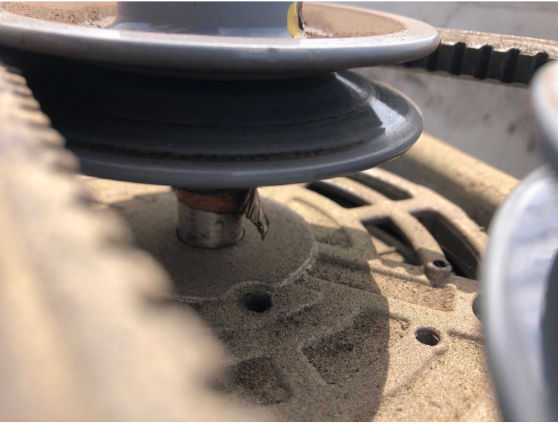
EF-H3 MOTOR PULLEY EDGES WORN.
