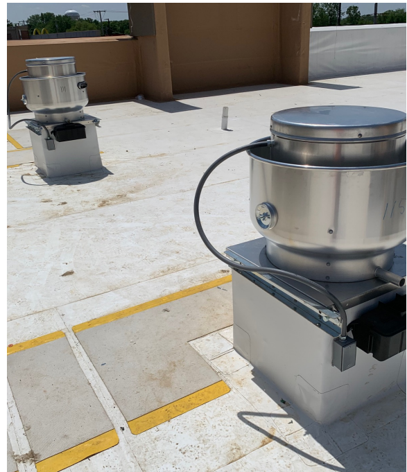
Grease Exhaust Fans
