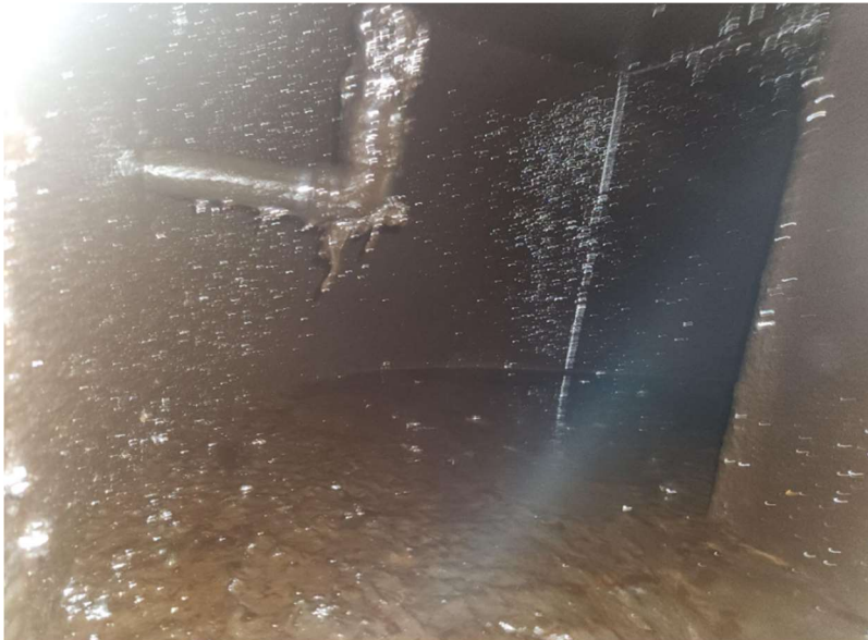
1 st floor inside the duct. Pools of grease
