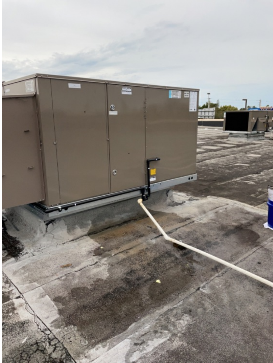
All 5 Sides of Installed Unit of RTU - Including Top with Condensor Fan Section. (4)
