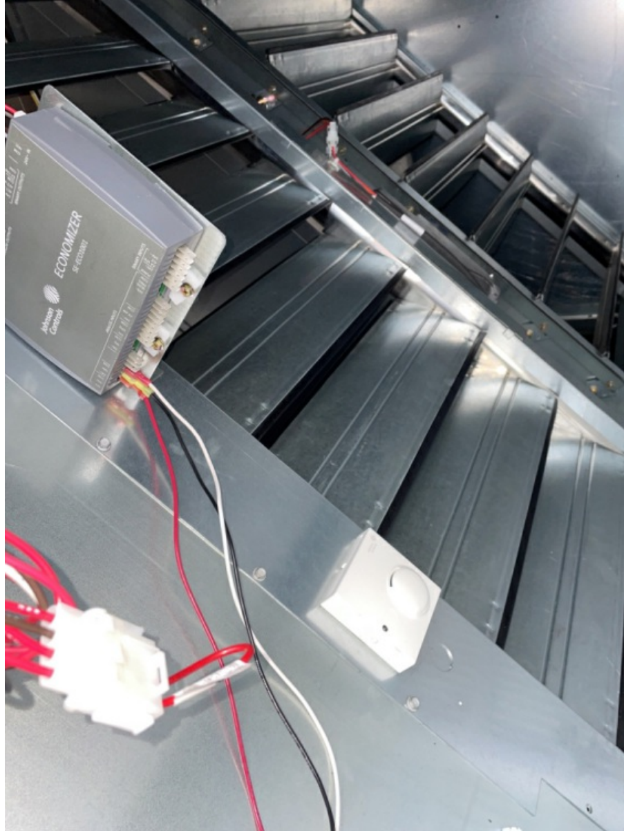
Installed RTU Economizer Photo (1)
