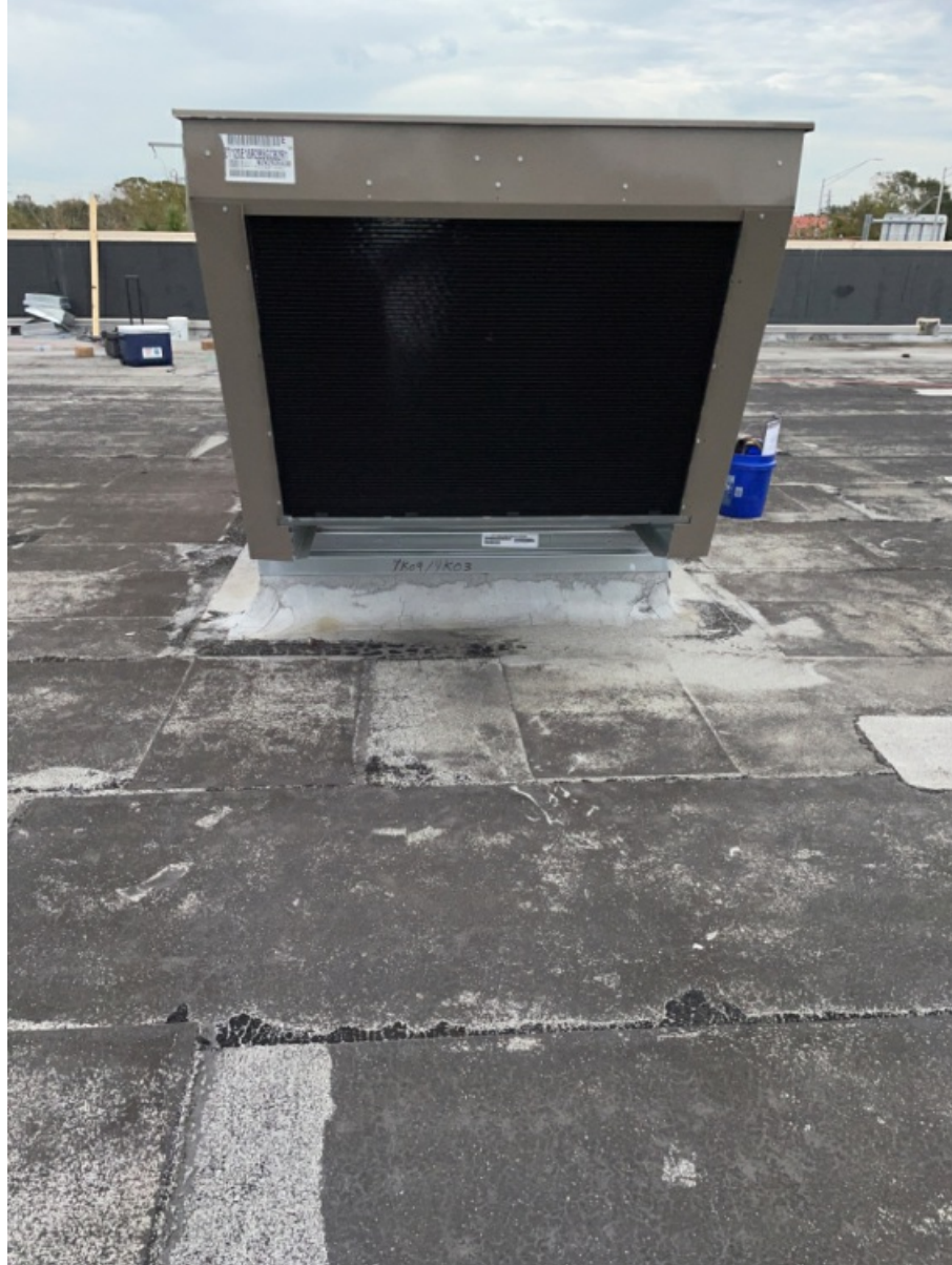
All 5 Sides of Installed Unit of RTU - Including Top with Condensator Fan Section. (1)
