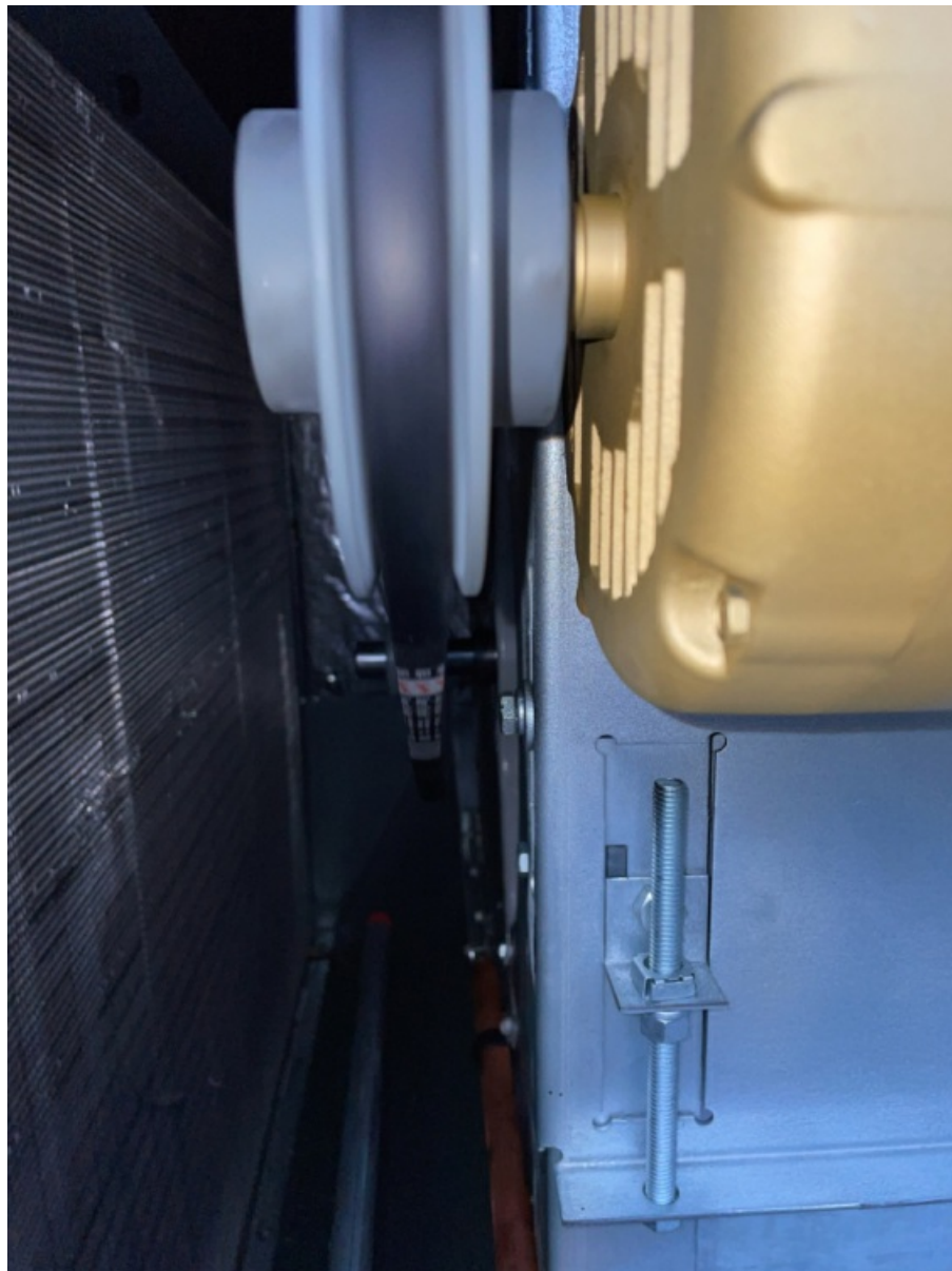
Alignment of RTU Drive Component Photo (1)
