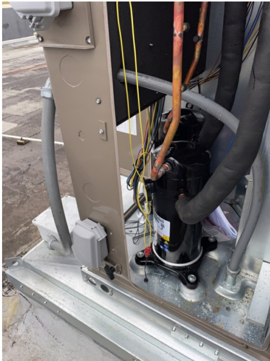
All RTU Field Power Wiring Photo (1)
