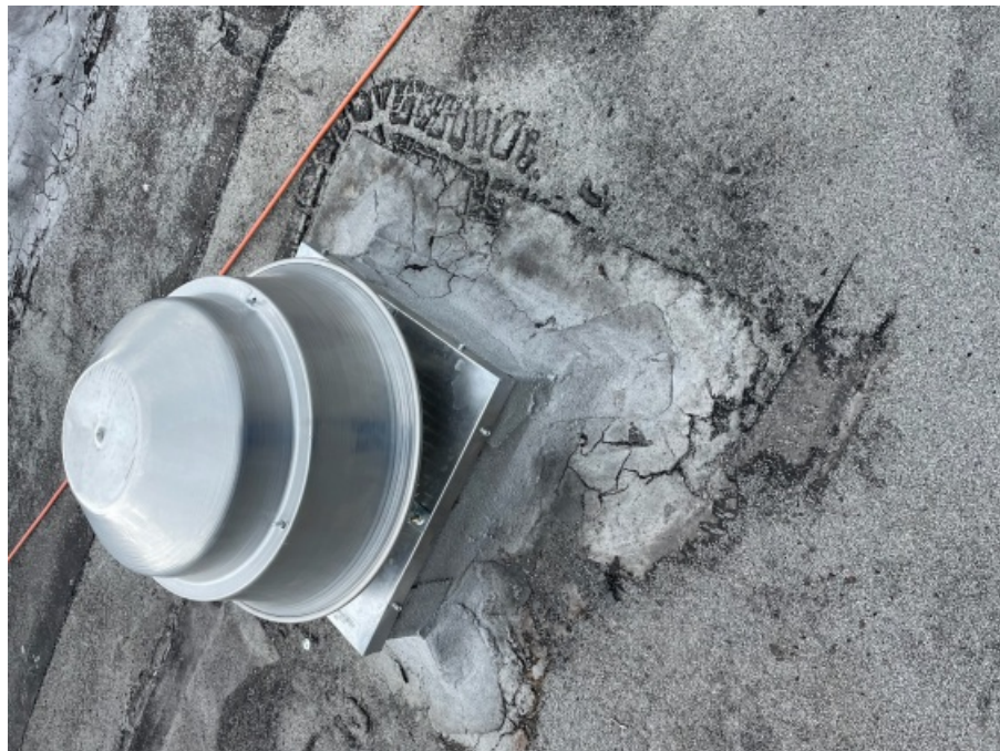
All 5 Sides of Installed Unit - Including Top (7)
