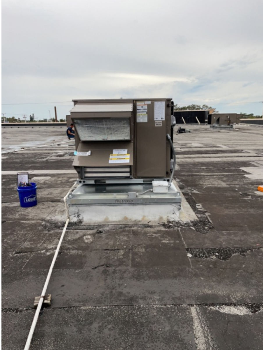
All 5 Sides of Installed Unit of RTU - Including Top with Condenser Fan Section. (3)
