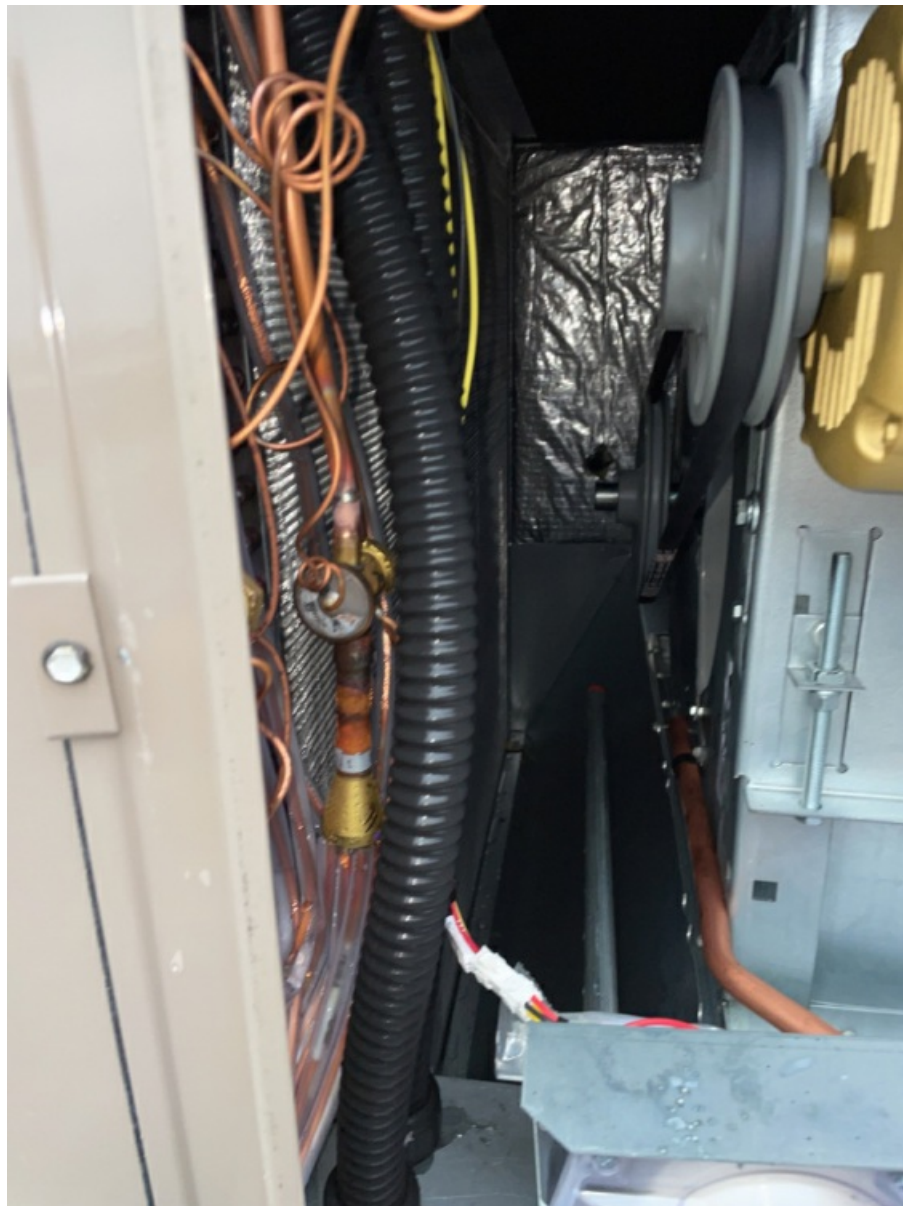
Interior Pictures of RTU Blower Section, Power / Control Section, Heat Section, Compressor Section. (1)
