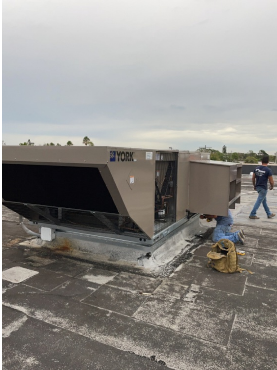
All 5 Sides of Installed Unit of RTU - Including Top with Condensor Fan Section. (3)
