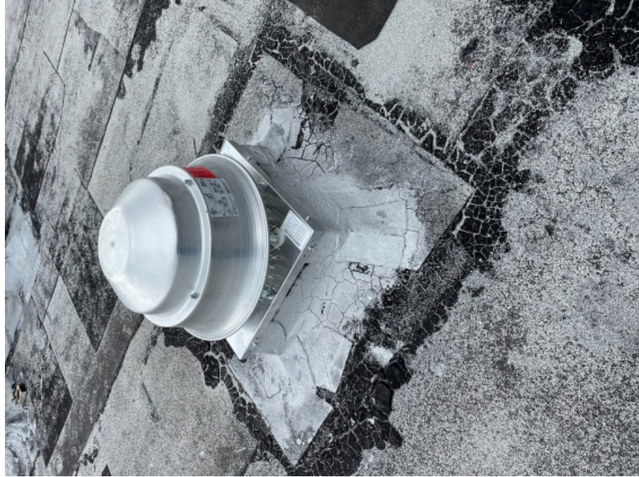
All 5 Sides of Installed Unit - Including Top (3)
