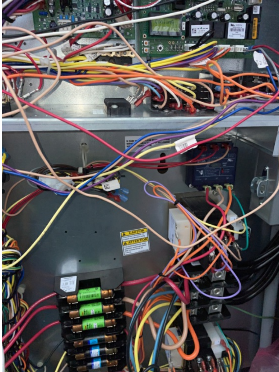
All RTU Field Control Wiring Photo (1)
