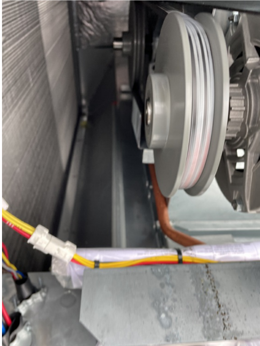
Alignment of RTU Drive Component Photo (1)
