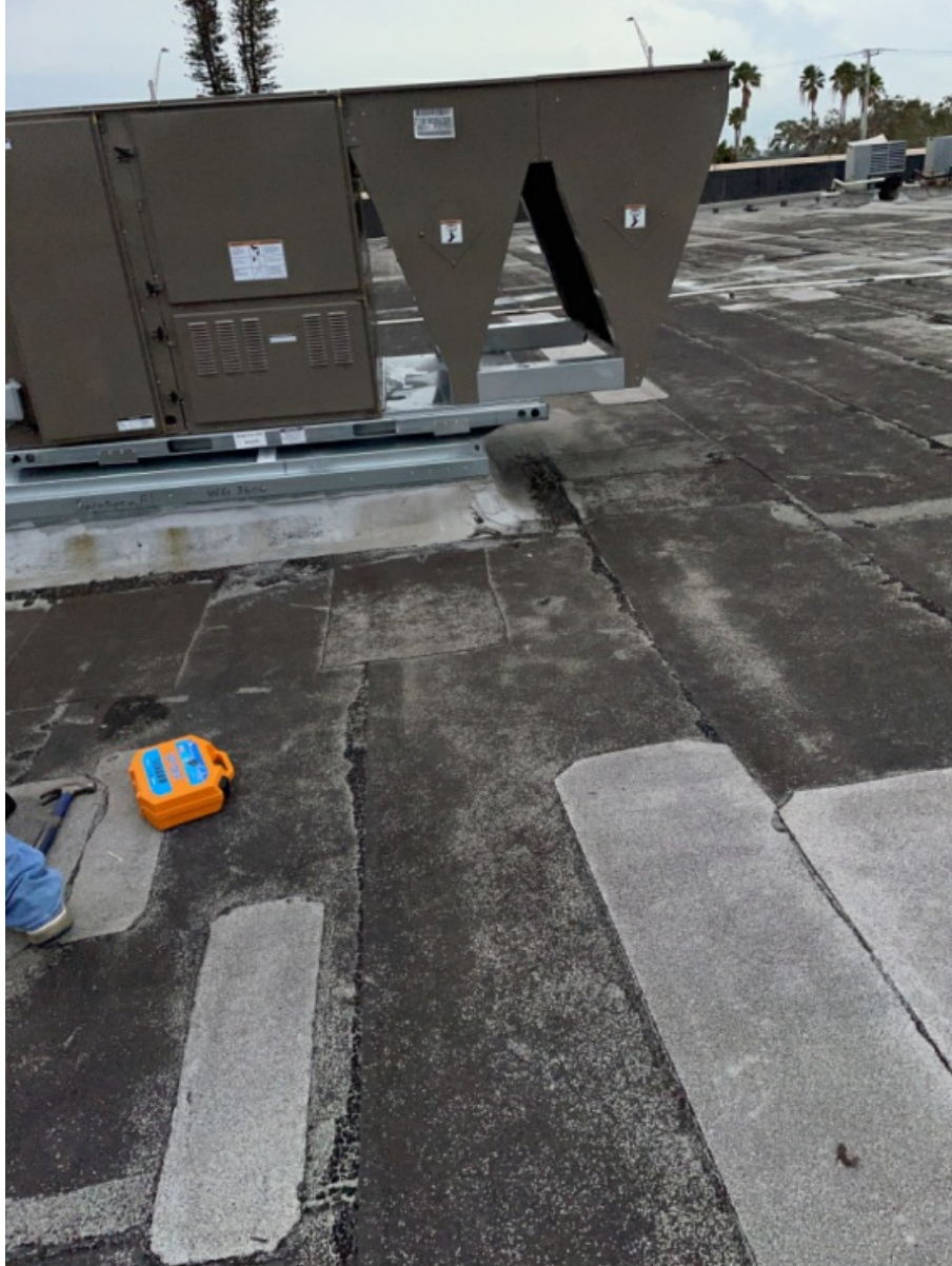
All 5 Sides of Installed Unit of RTU - Including Top with Condensor Fan Section. (4)
