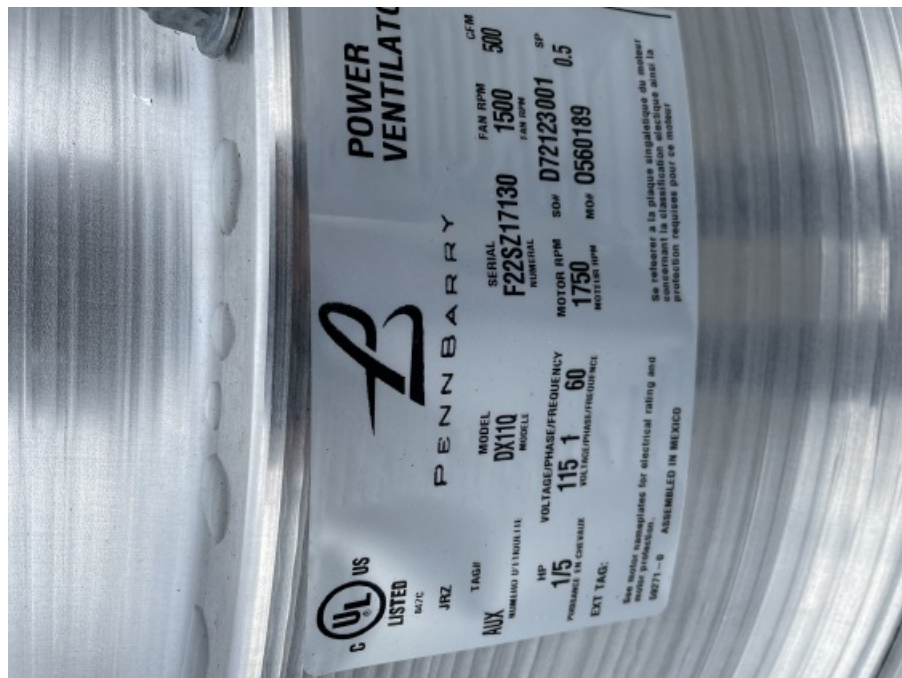
Exhaust Fan Unit Name Plate Photo (2)
