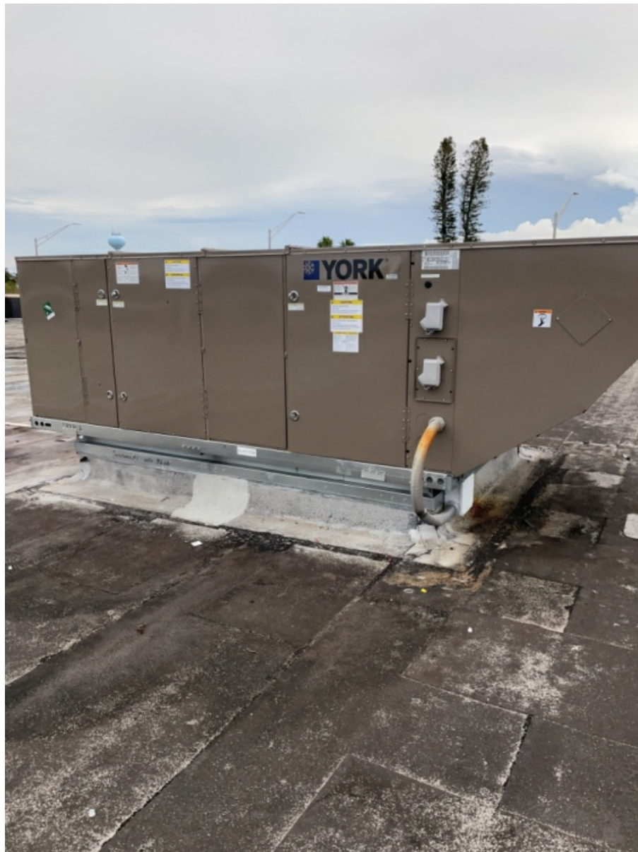
All 5 Sides of Installed Unit of RTU - Including Top with Condenser Fan Section. (1)
