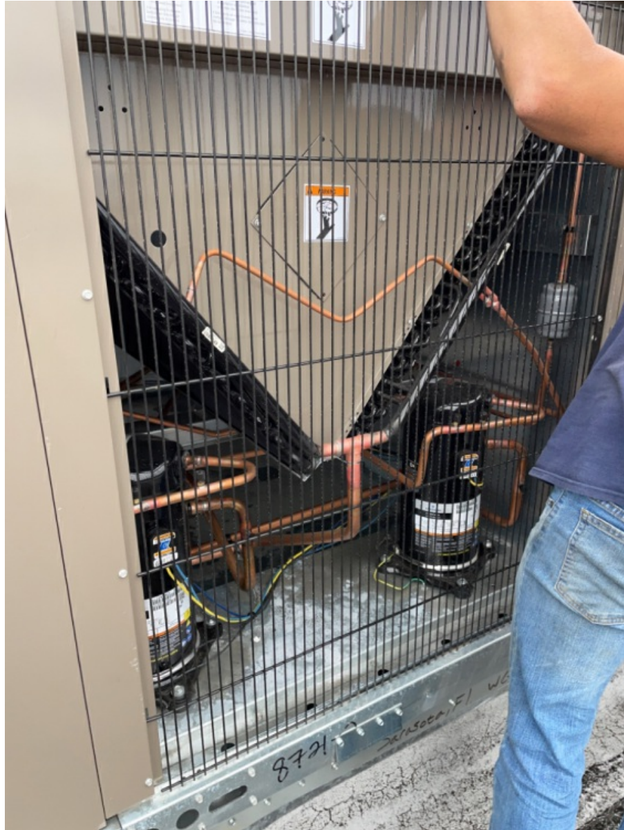
Interior Pictures of RTU Blower Section, Power / Control Section, Heat Section, Compressor Section. (3)
