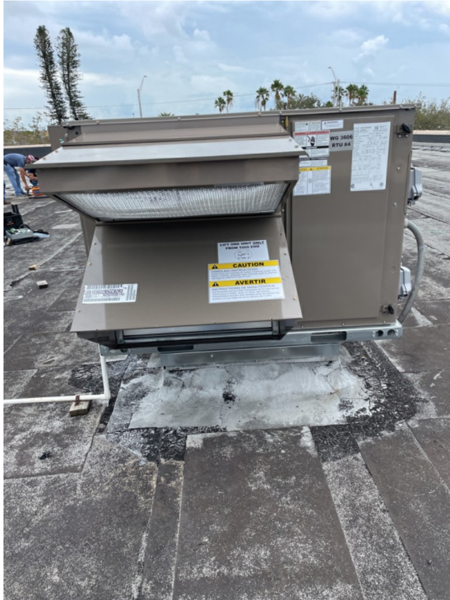
All 5 Sides of Installed Unit of RTU - Including Top with Condenser Fan Section. (4)
