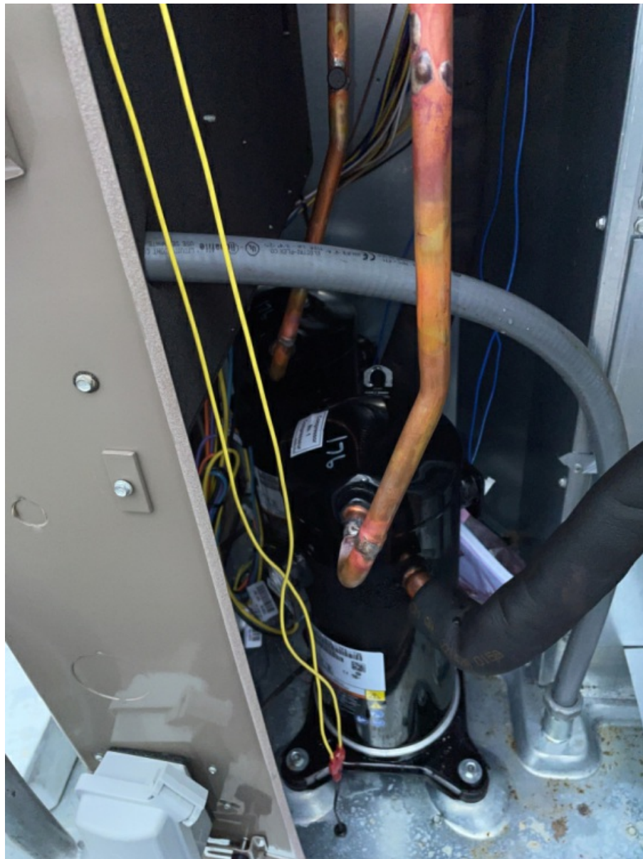
Interior Pictures of RTU Blower Section, Power / Control Section, Heat Section, Compressor Section. (2)
