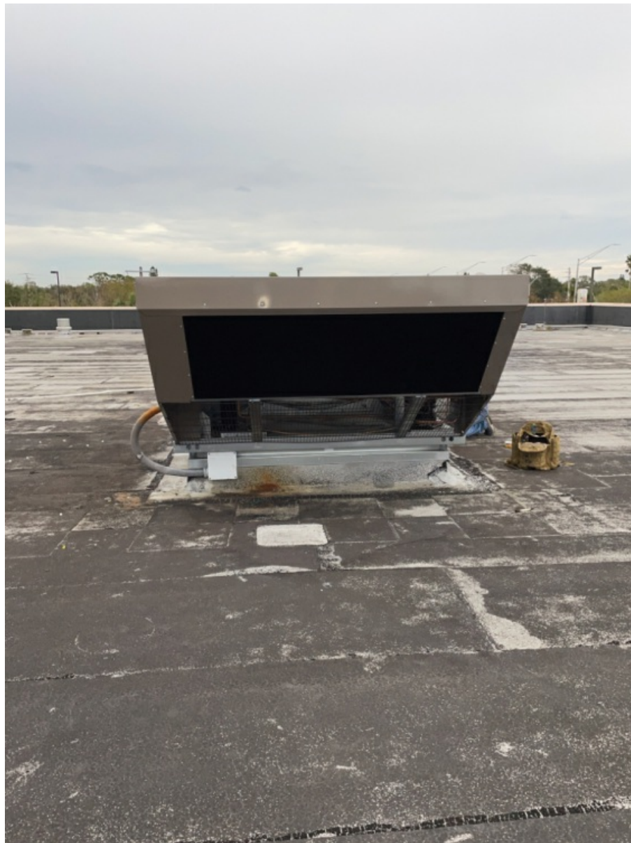
All 5 Sides of Installed Unit of RTU - Including Top with Condensator Fan Section. (2)
