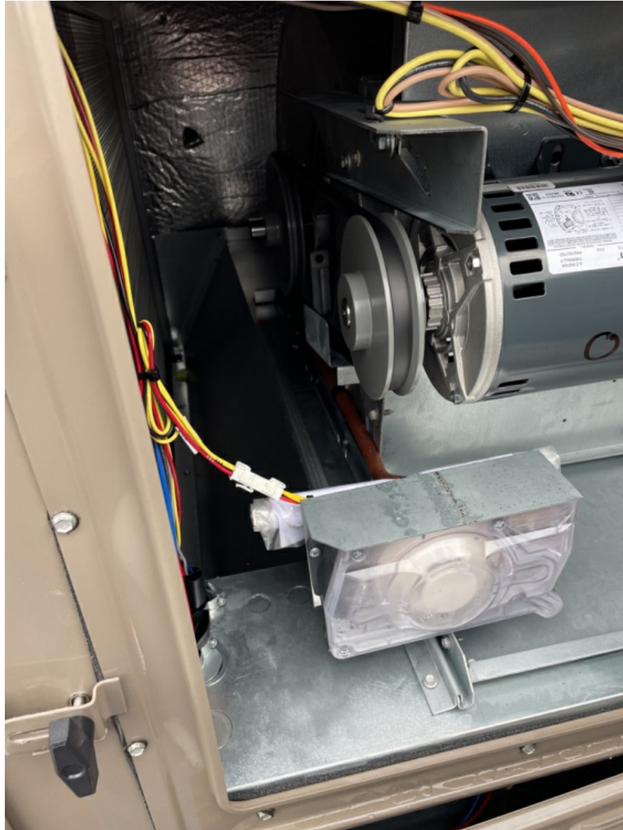
Interior Pictures of RTU Blower Section, Power / Control Section, Heat Section, Compressor Section. (1)
