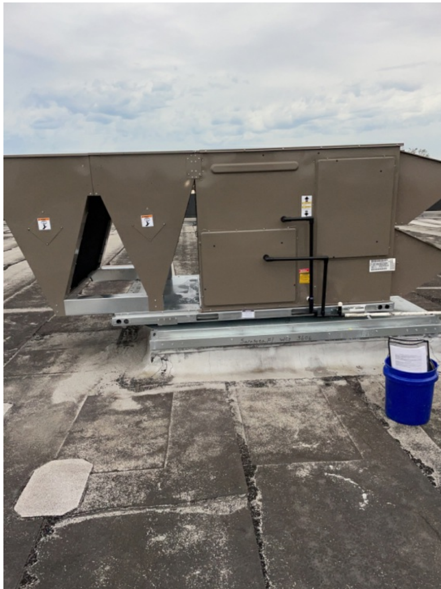
All 5 Sides of Installed Unit of RTU - Including Top with Condensator Fan Section. (2)
