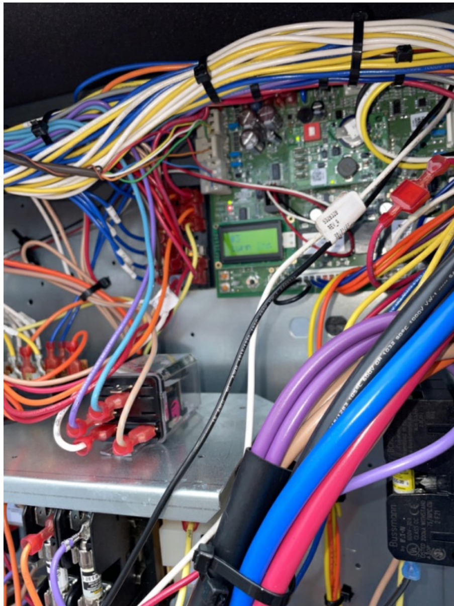
All RTU Field Control Wiring Photo (1)
