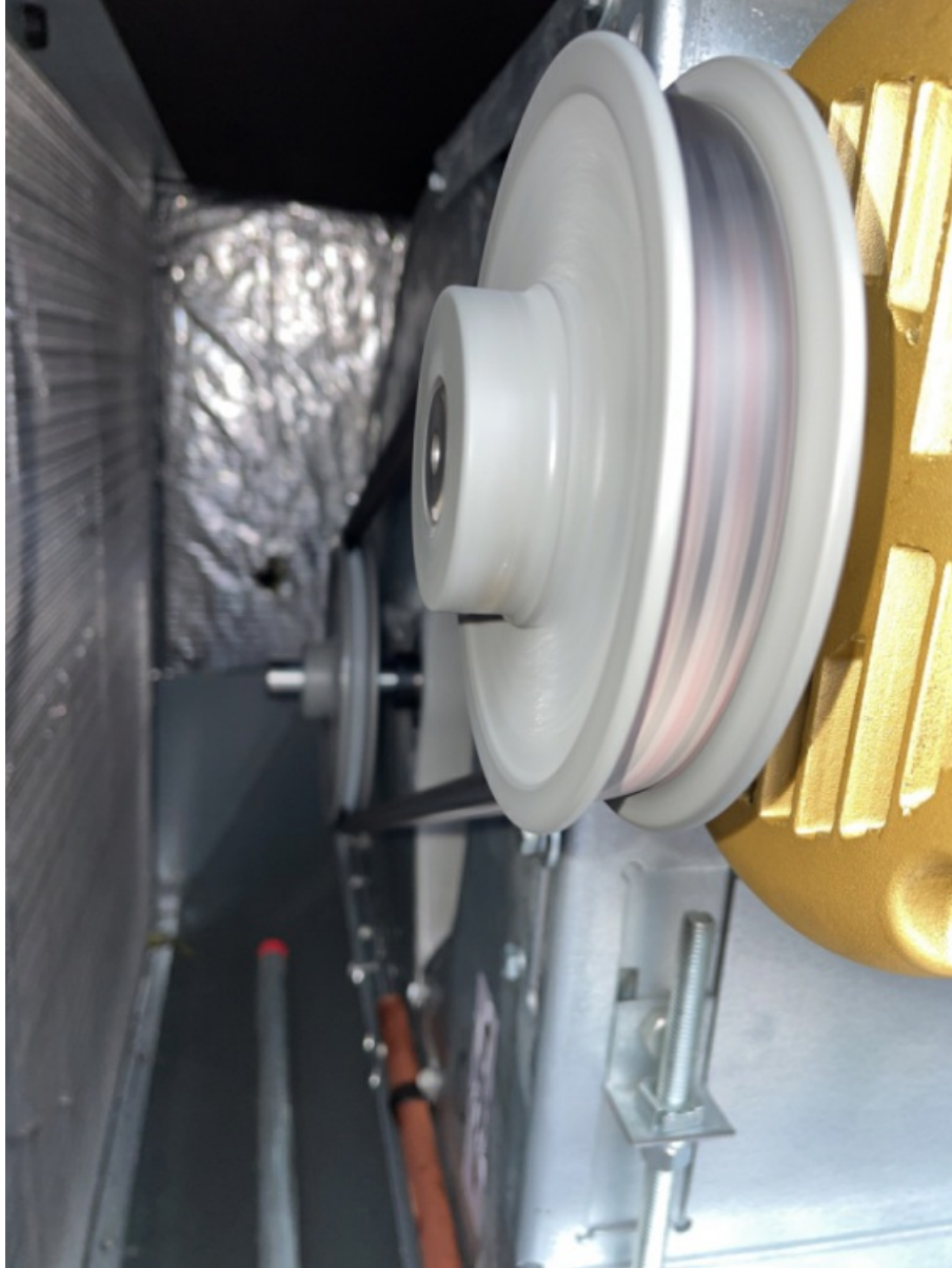
Alignment of Blower Pulley Key Flush with End of Blower Shaft (1)
