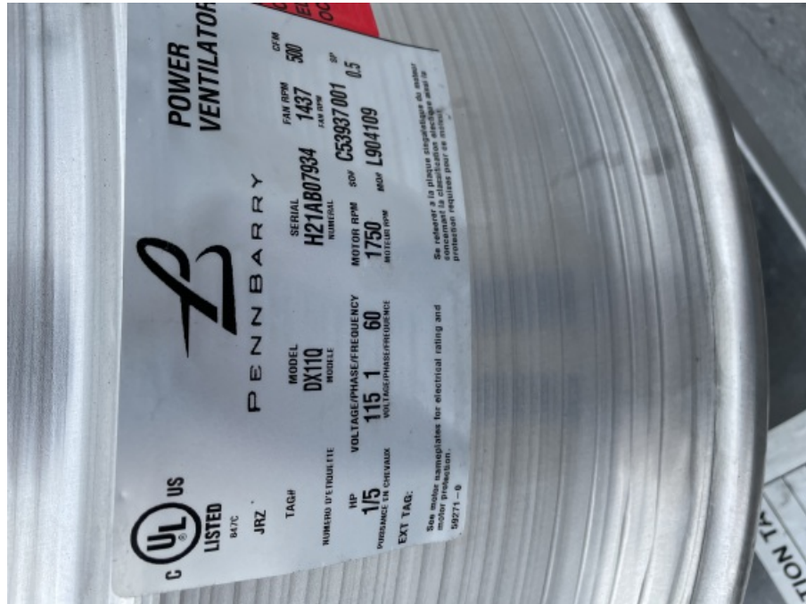
Exhaust Fan Unit Name Plate Photo (4)
