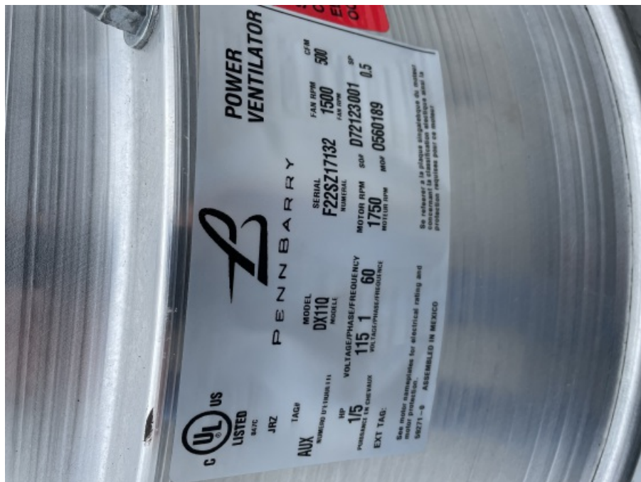
Exhaust Fan Unit Name Plate Photo (6)
