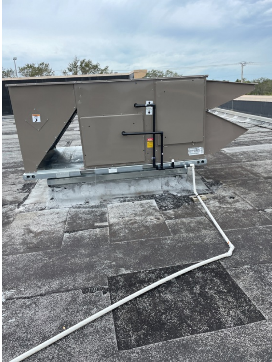
All 5 Sides of Installed Unit of RTU - Including Top with Condenser Fan Section. (3)
