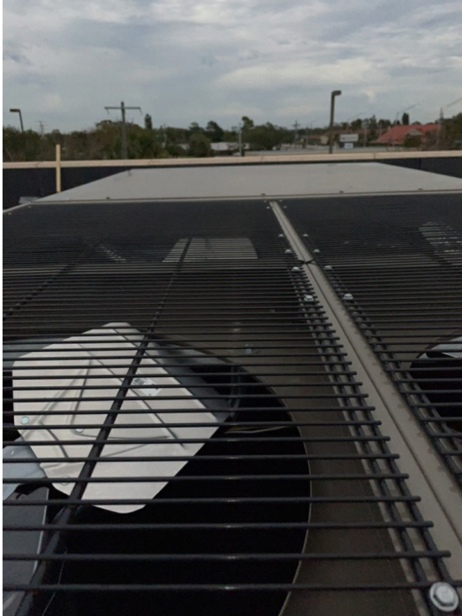
All 5 Sides of Installed Unit of RTU - Including Top with Condensor Fan Section. (5)
