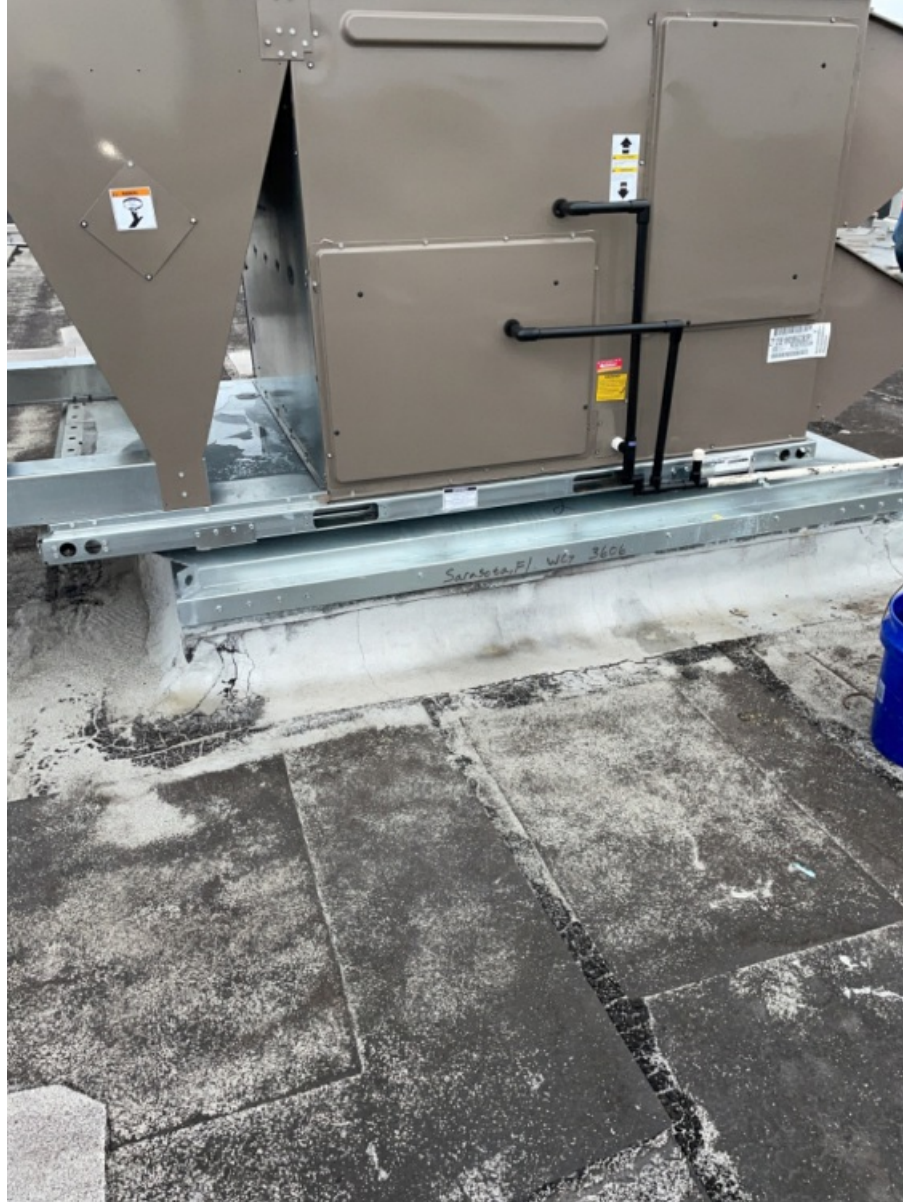
Pictures of RTU Unit Mounting to Roof Curb / Adapter Curb Showing Proper Alignment and Sealing. (1)
