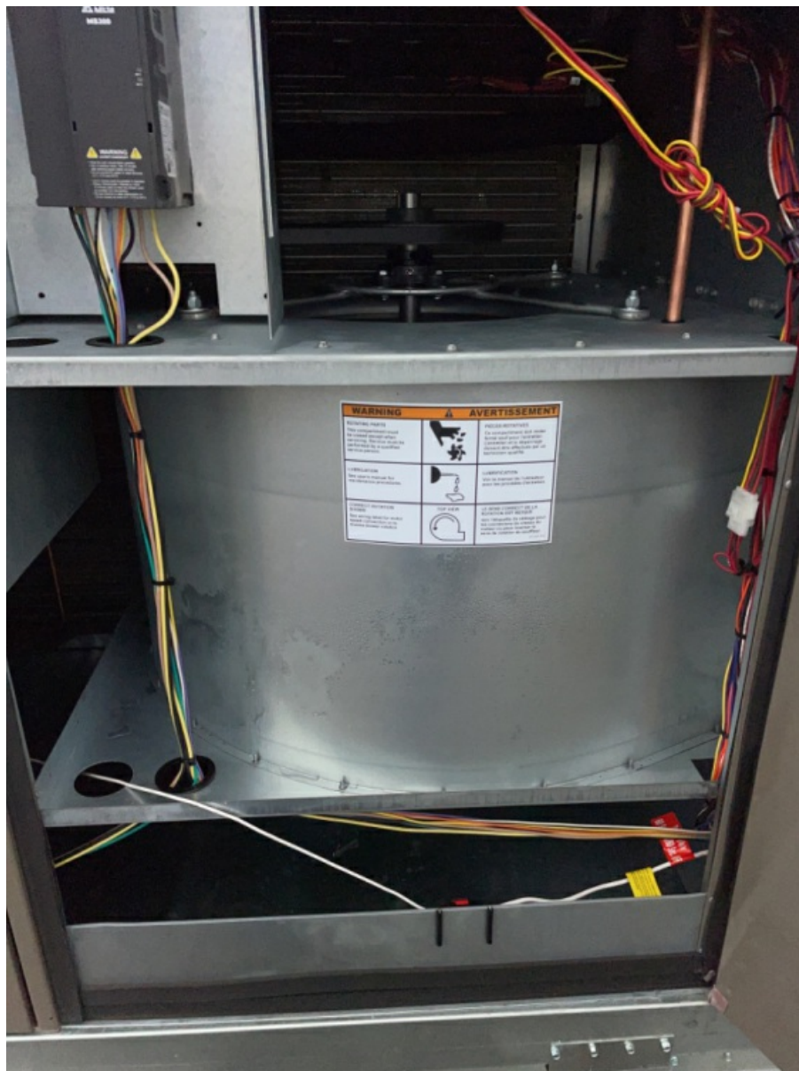
Interior Pictures of RTU Blower Section, Power / Control Section, Heat Section, Compressor Section. (1)
