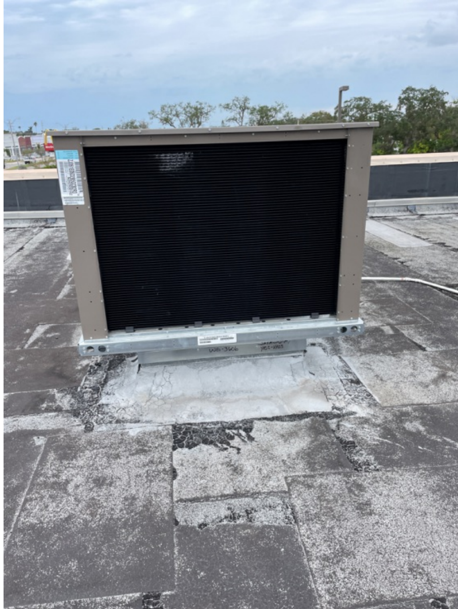
All 5 Sides of Installed Unit of RTU - Including Top with Condenser Fan Section. (2)
