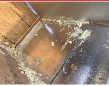
AHU-A R/A BOX Not sealed properly
