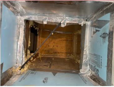
AHU-A R/A BOX Not sealed properly
