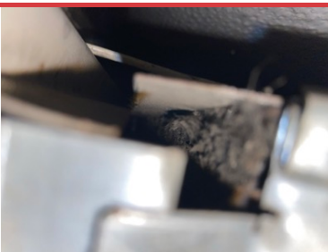
AHU-A. S/A PLENUM Not sealed properly
