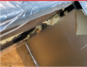
AHU-A. R/A BOX Not sealed properly
