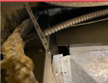
AHU-A. SUPPLY AIR PLENUM Not sealed properly
