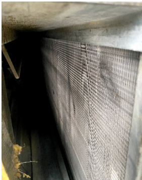
RTU-3 (KITCHEN) DIRTY EVAPORATOR
