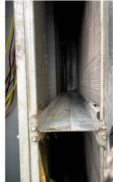
RTU-3 (KITCHEN) CLEAN EVAPORATOR
