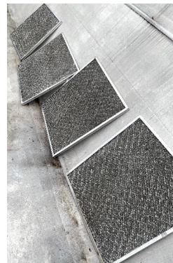
RTU-2 (DINING) CLEAN OUTSIDE AIR FILTERS
