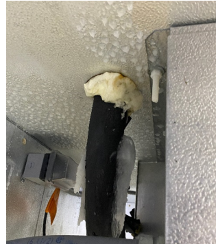
WALK-IN FREEZER ICE BUILD UP ON PENETRATION PIPE
