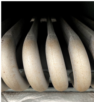
RTU-3 (KITCHEN) BURNER TUBE INSPECTION
