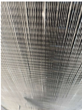
RTU-3 (DINING/ORDERING) DIRTY CONDENSER
