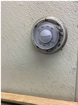
FURNACE THERMOSTAT OLD RECOMMEND REPLACEMENT
