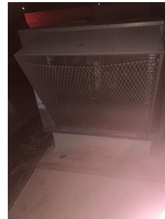
RTU-3 BIRD CAGE IS DAMAGED AND HANGING OFF UNIT
