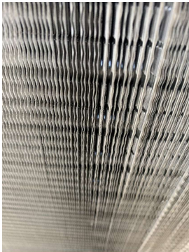
RTU-4 (KITCHEN) DIRTY CONDENSER
